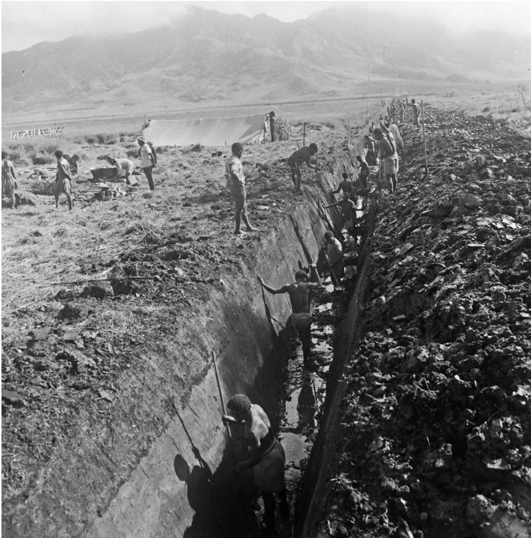
Figure 6.16 Digging the eastern boundary drain of Kuk Station in the course of the development of the drain and road network shown in Figure 6.1.
