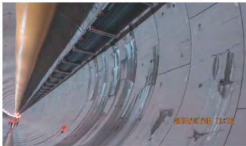
Figure 3. Photo from a typical bad zone with multiple cracks & leakage.
