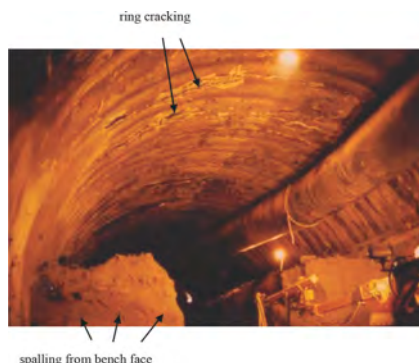
Figure 6. Last glimpse into the tunnel before collapse at chainage 109-111.
