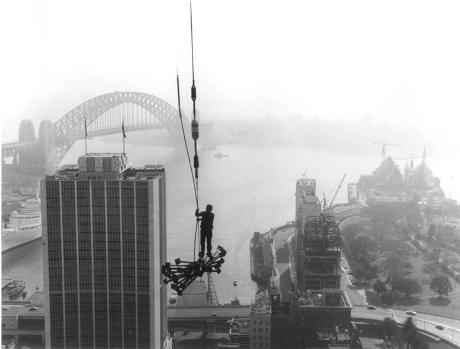
Figure 2.2: Things had not changed much by 1965. This photo, taken by Valentin Sowada, shows Lance Shelton, known to other BLs as ‘Blackie’ or ‘Sooty’. He was an Aboriginal member of the NSW BLF riding on a load in the construction of the State Office Block. The photograph is known as ‘The Rigger, Sydney c. 1965’. This photograph was held in Joe Owens private collection, and he explained that this image was widely circulated among NSW BLF members in the 1960s and 1970s, particularly among those, like Kevin and Joe, who had worked as dogmen.
