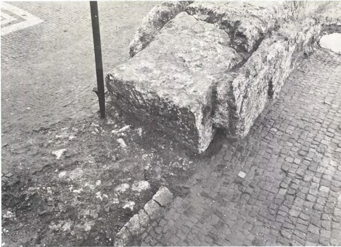
a. Insula XXI, Building 2: doorway of Room 4 from Corridor 2 showing quarter-round moulding, emplacement of door-frame, and cracked wall over decayed wooden threshold (pp. 163-4).
