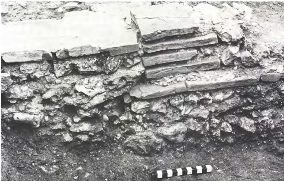
b. Insula XXII, Building 1: junction of Walls 2 and 3 from the south-east. Wall 3 (left) abuts the tiled quoin of Wall 2 which itself oversails Wall 1 (pp. 184, 187).
