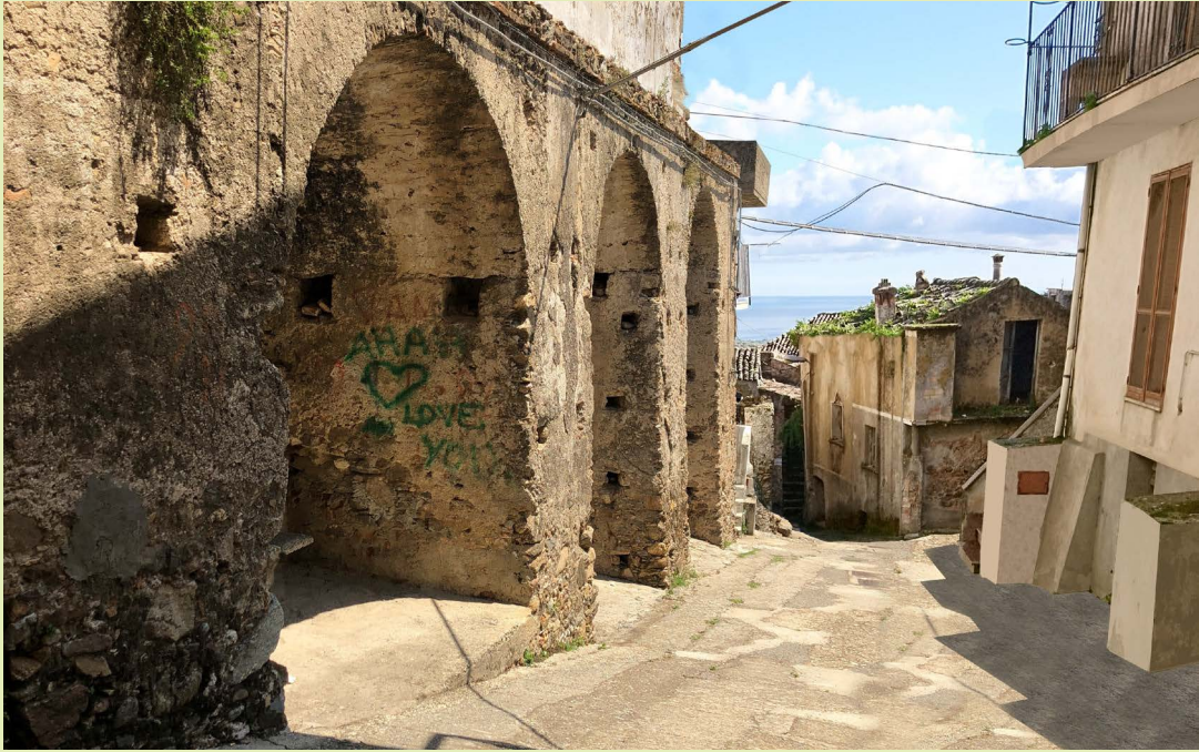
FIGURE III.4.4 The existing entrance to medieval Borgo. Photo by Rob Wills, Emma Kingman, James Anderson.
