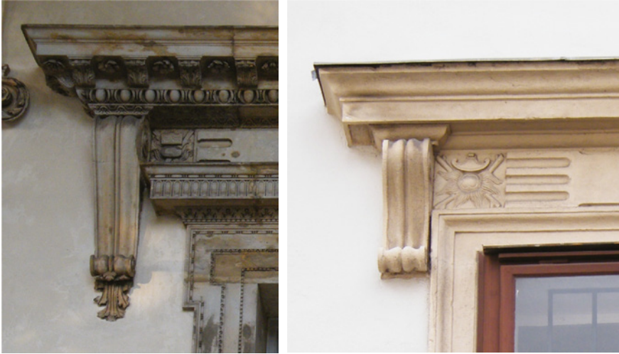
FIGURES 5.79–5.80 Lintel and entablature of a window frame of Queen Anna's Summer Palace, ca 1540–1545, compared to the Lintel and entablature of a window frame of the Schweizerische Trakt of the Hofburg, Vienna, ca 1553.
