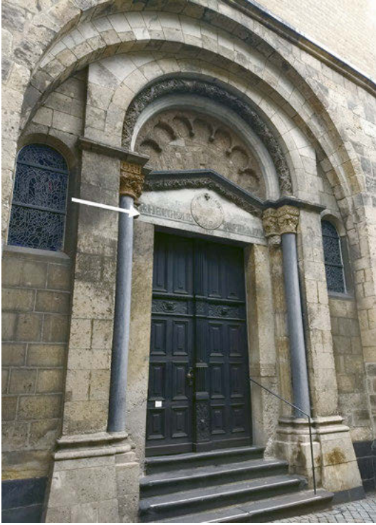
Figure 48: Floodmarks at the portal of St. Maria in Lyskirchen, Cologne. This church shows two floodmarks, one above the door, marked by a line, and one to the right of the entrance with a line indicating the height of the flood. The water reached approximately 3.50 meters above street level.
