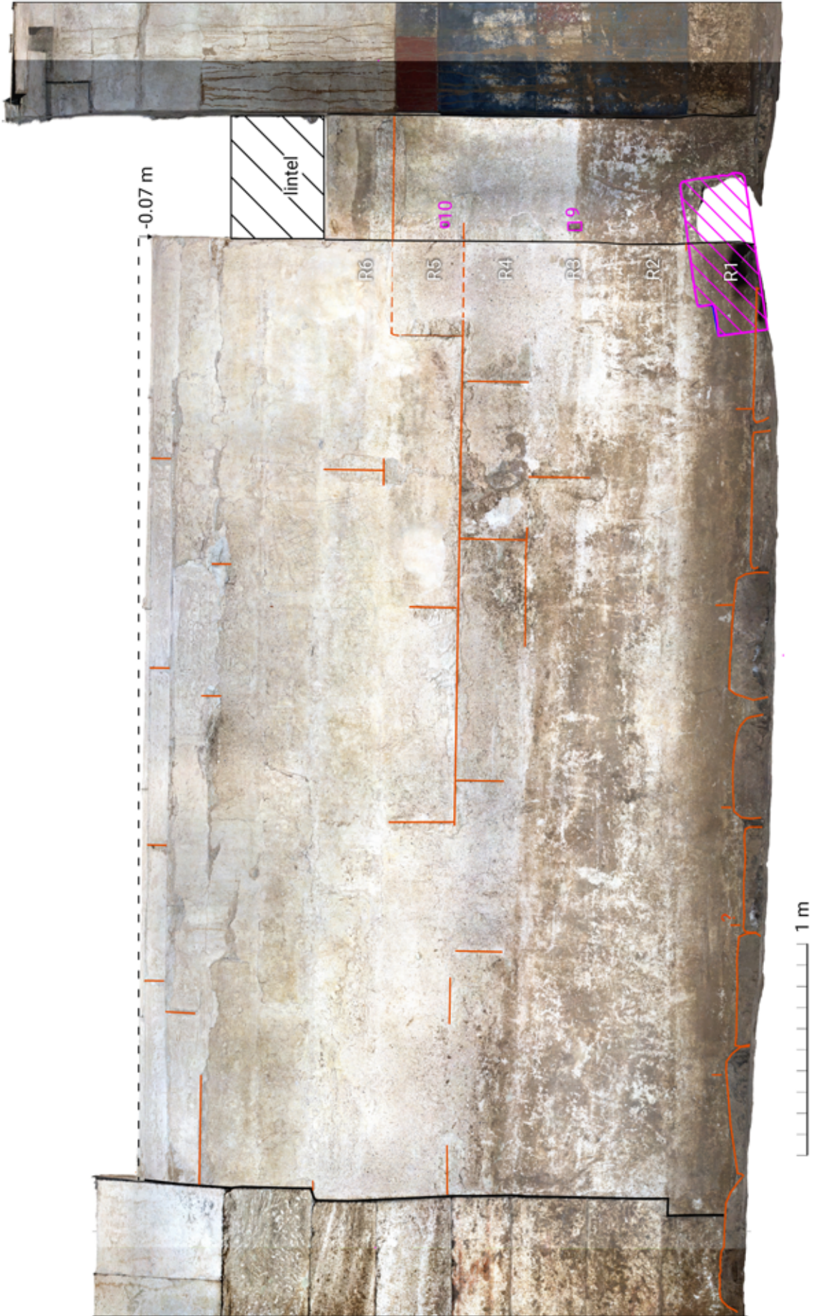
Figure 127. Dromos I , orthophoto of the southern wall; orange lines – plinths and ashlar joins visible in the areas where the plaster fell.
