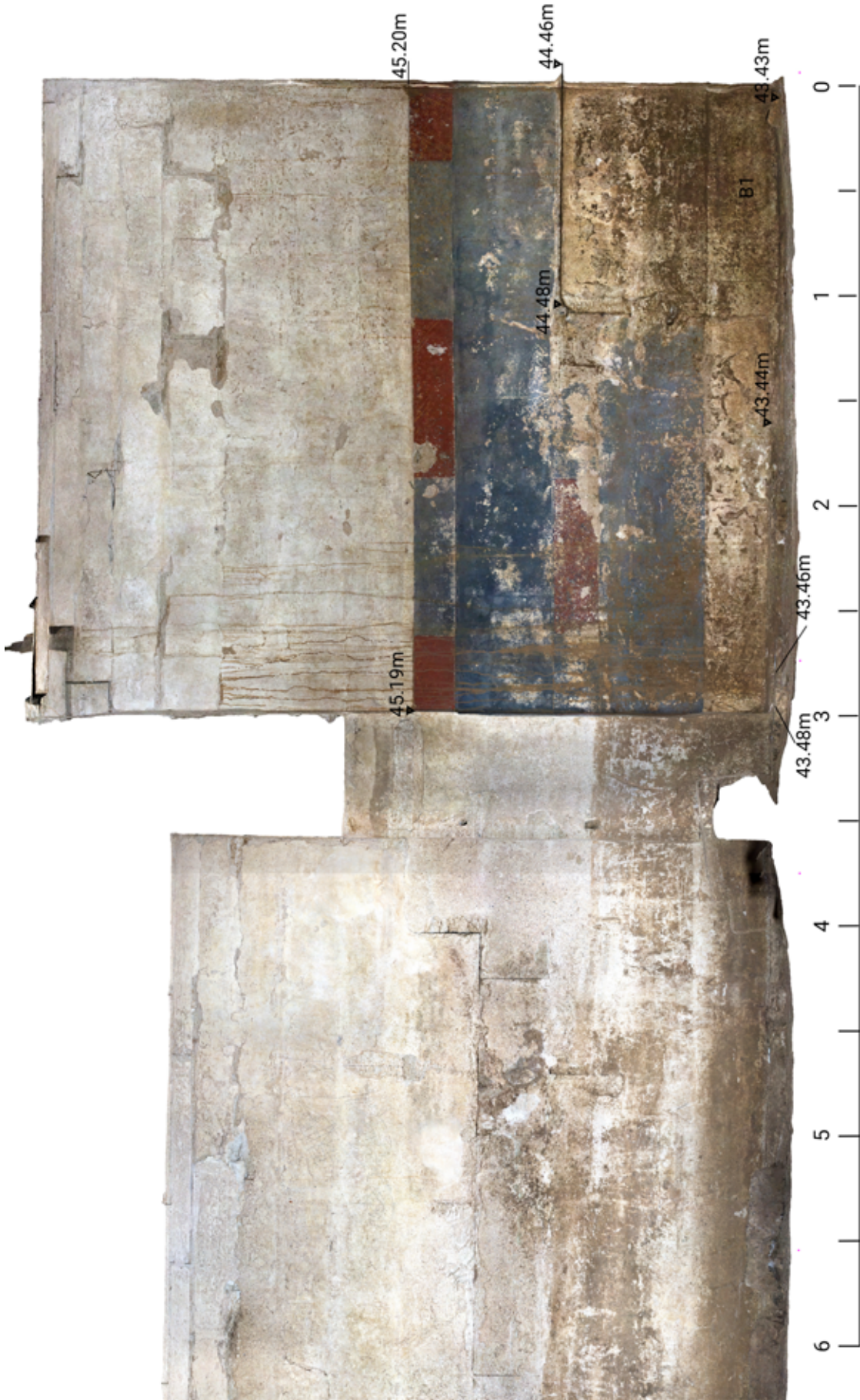
Figure 97. Southern wall of the funerary chamber and part of dromos I, absolute elevations.
