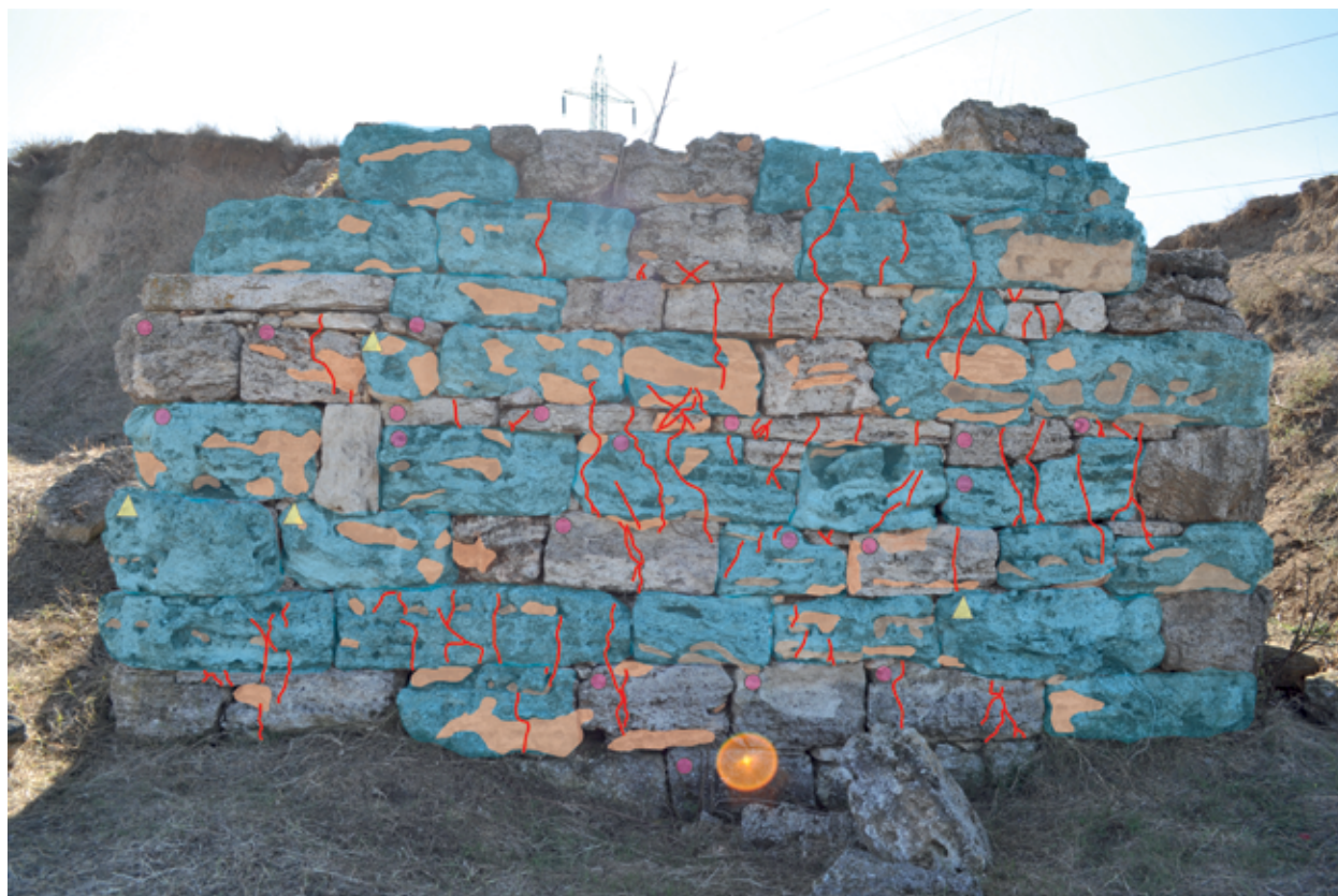
Cracks Alveolization Limonitization Shell-limestone Micritic limestone
