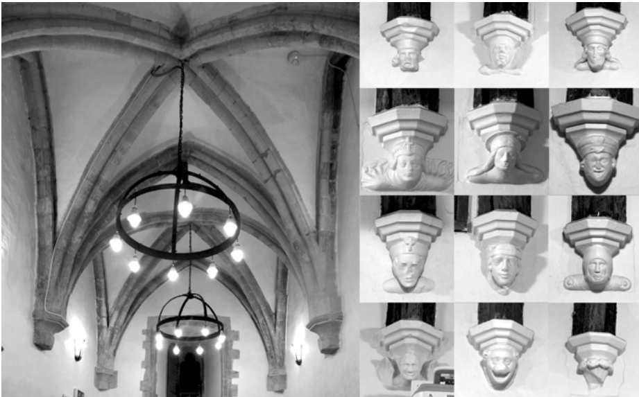
Fig. 4.6: Structural evidence thought to pre-date the 1362 storm at St Albans. Left: Rib vaults in one of the ground floor chambers. Right: Decorated corbels now located inside chambers on the second floor of the gatehouse of St Albans Abbey. Photographs by the author.
