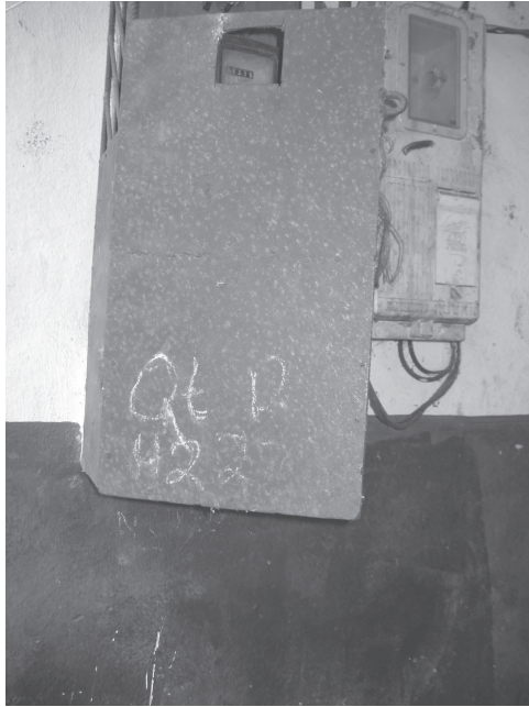
Figure 2.74 Electricity cabinet, Mutengene, Cameroon.
