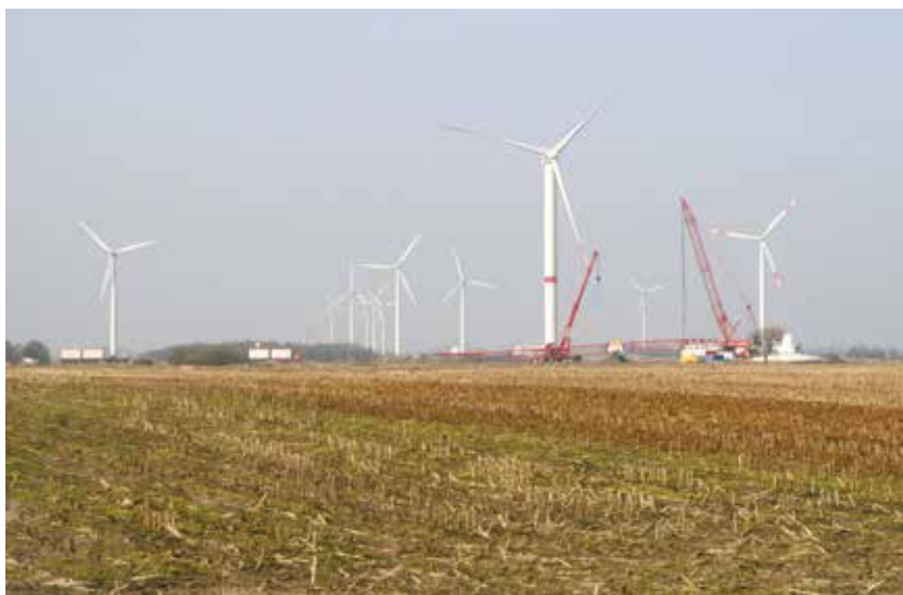
Figure 18.2 The erection of wind power plants has repercussions for the landscape that go far beyond the actual location of the plants, as demonstrated by the example in the northern part of the district of Nordfriesland: it is accompanied by the construction of infrastructure, trenches for cables, electric power transformation stations and high-voltage power lines.
