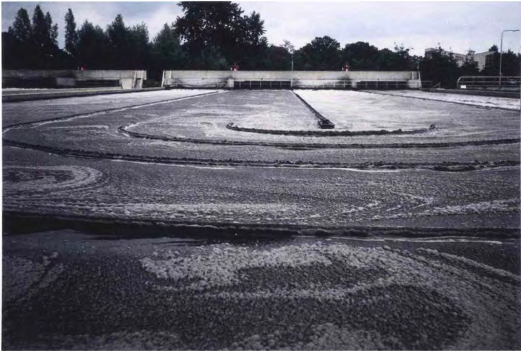
Figure 84 The aeration tank is completely covered by scum.
