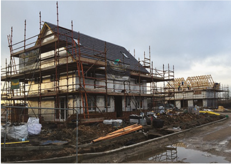
Figure 13.10 The homes on the first Potton site near St Helens are now coming out of the ground (© Buildstore)
