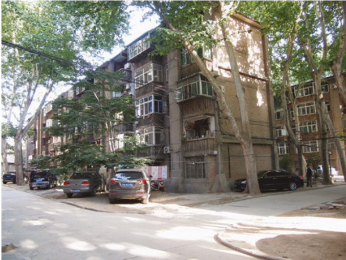
Figure 1.4 The staff housing in No. 1 Village, Xi'an Jiaotong University. This part was constructed in the late 1970s but it deteriorated quite significantly as shown in the photo. Taken in 2016.
