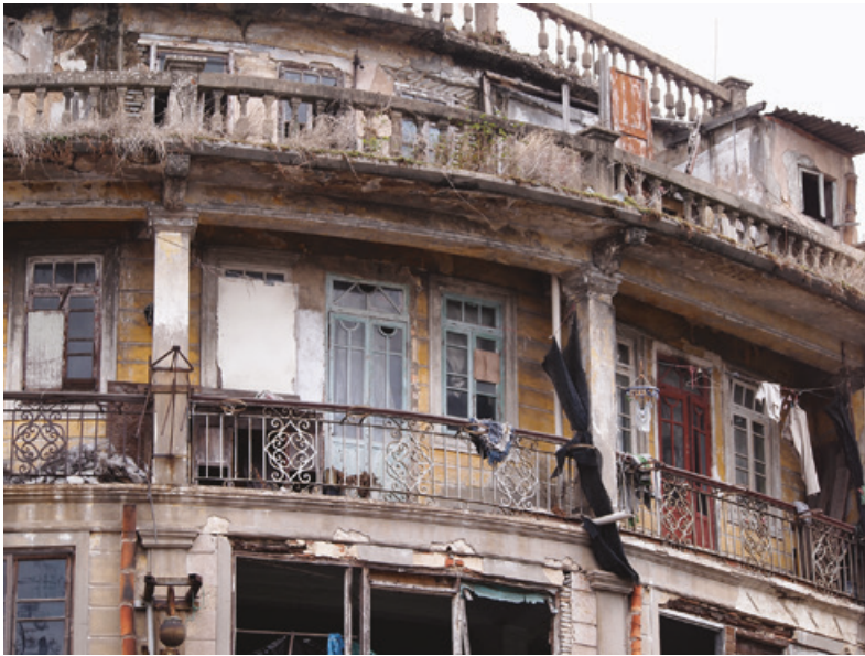
Figure 5.2 The dilapidated central area near the ‘Little Park’ in Shantou, showing a different trajectory from Xintiandi. Inner-city decline is rather rare in China. Taken in 2014.
