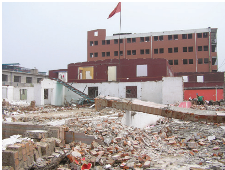
Figure 3.10 The demolition of Tangjialing village, Beijing. The demolition and redevelopment were rather swiftly completed owing to the programme of affordable housing provision in Beijing, which is largely for registered Beijing residents. Taken in 2010.
