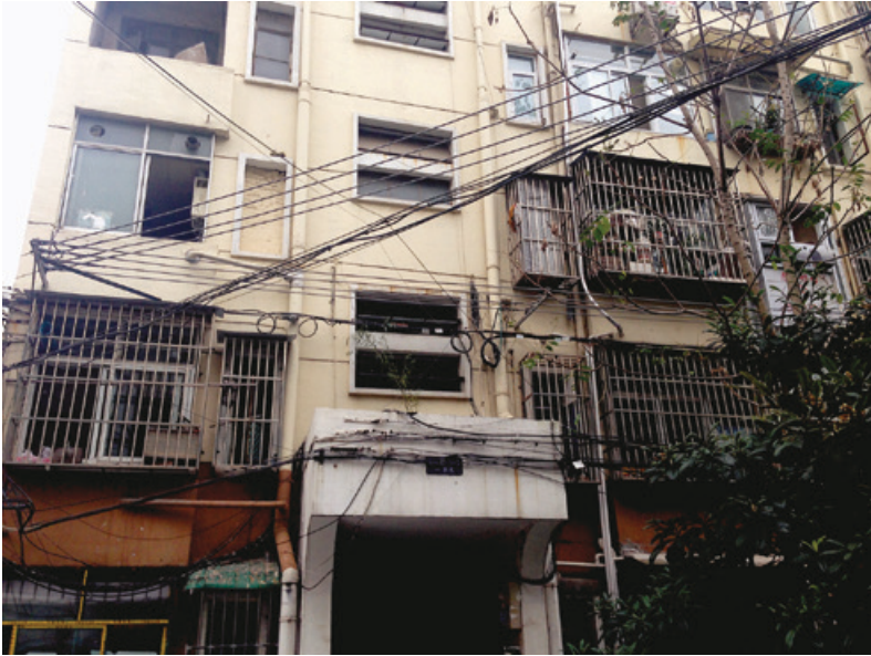
Figure 2.10 Signs of deterioration in the Fifth Village, Nanjing. The original internal sewer pipes were blocked and an external duct had to be built. Housing privatisation does not enhance estate maintenance but rather has led to the withdrawal of workplaces' responsibility for maintenance. Taken in 2014.
