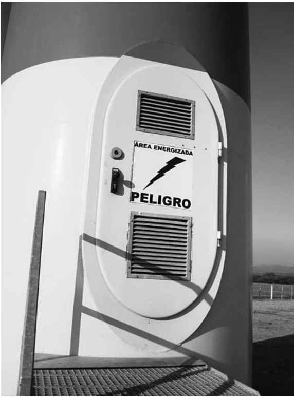
FIGURE 1.6. Turbine tower with DANGER sign
