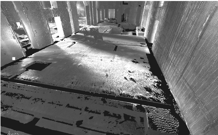
Figure 6.8: Snapshot of the ruined part of the bunker in the generated 3D-model.
