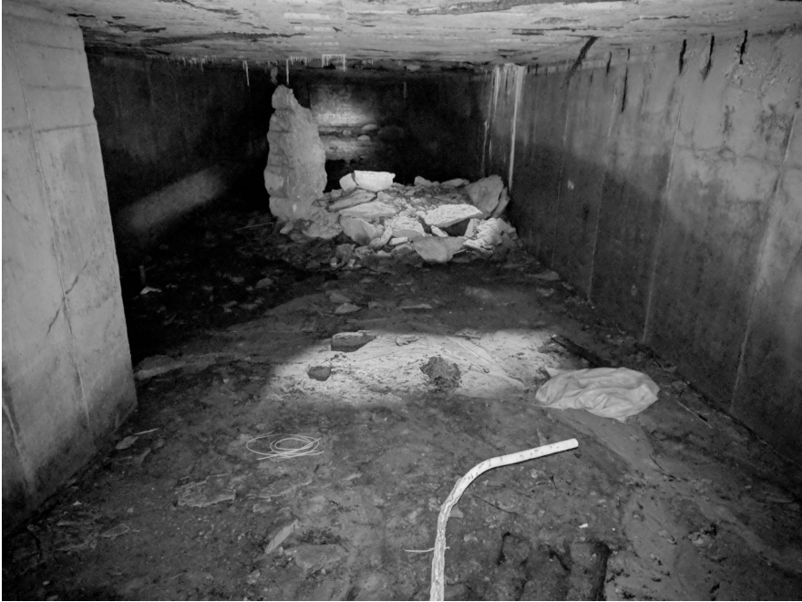
Figure 6.2: Underground tunnel with gravel from collapsed ceiling.
