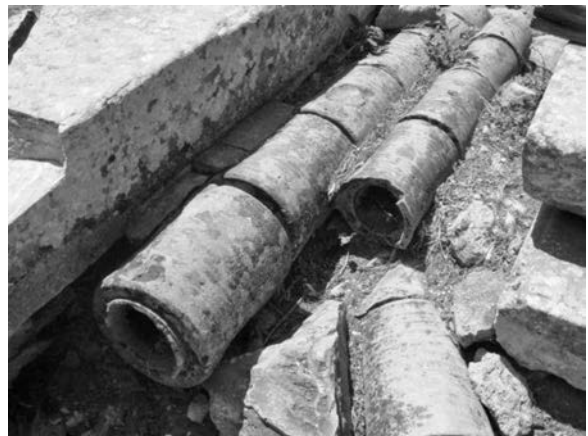
Figure 13.26 Two terracotta pipelines observed near the Tomb built for Androclus in Ephesus
