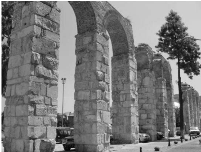
Figure 13.3 Part of a bridge in the Selinus aqueduct delivering water to Ephesus
