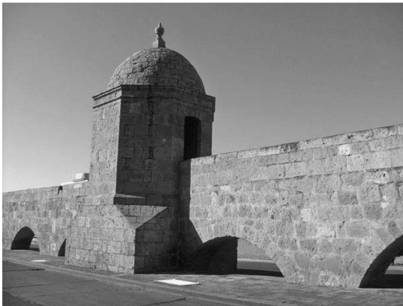
Figure 15.17 Aqueduct in the city of Morelia, Michoacan, Mexico (Source: Wikipedia Commons, in Public Domain)
