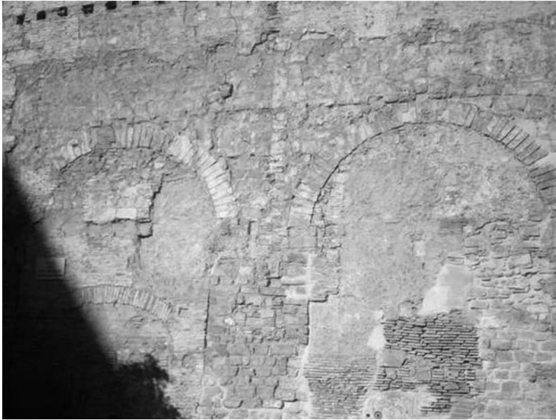
Figure 19.3 Badly preserved arches of the Roman aqueduct, Barcelona (with permission of M. Salgot)
