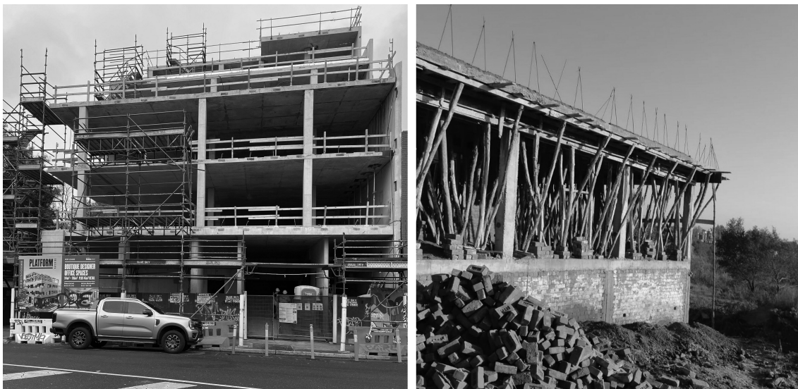
FIGURE 11.1 Residential construction in Melbourne and Islamabad in November 2022. There are obvious differences in practices.
