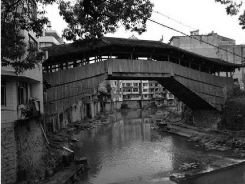
Figure 11.3 Xue Hamlet Bridge (destroyed by a flood in September 2016)
