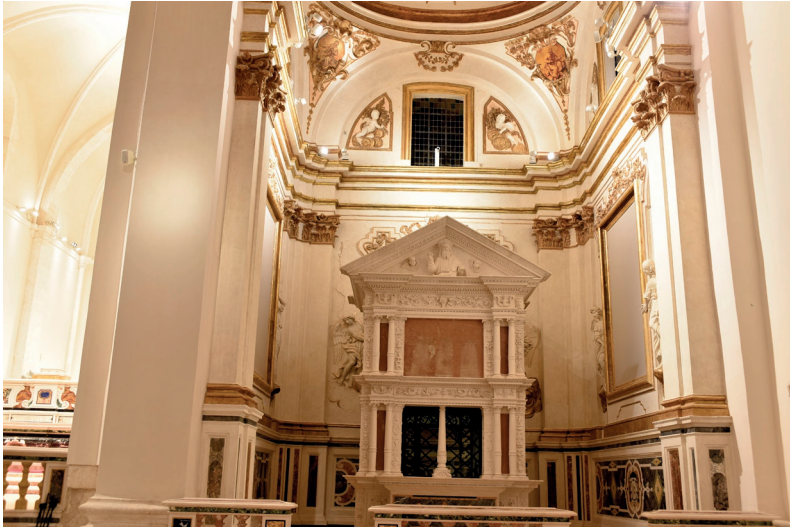
Figure 1.5 Santa Maria di Collemaggio: the discovery of the original gildings in the Celestine Chapel.
