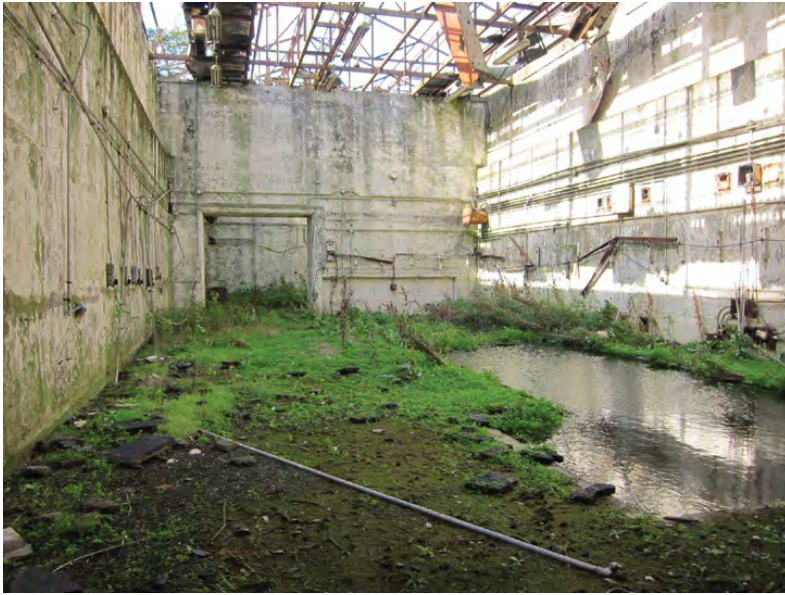
Figure 23.6 A community of plants that has established in one of the AWRE structures since the National Trust's acquisition in the 1990s (photograph by Caitlin DeSilvey).
