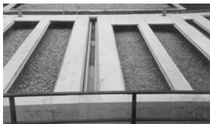
Figure 27.4. Anaerobic filter after UASB reactor (source: Ipatinga WWTP, COPASA, Brazil)
