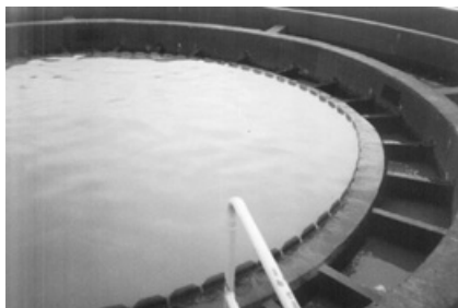
Figure 27.16. Influent distribution structure in a circular reactor (source: Nova Vista WWTP, SAAE Itabira, Minas Gerais, Brazil)
