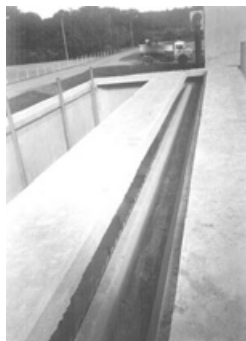
Figure 27.6. Effluent collection launder on the top of an anaerobic filter (Ipatinga WWTP, COPASA, Brazil)
