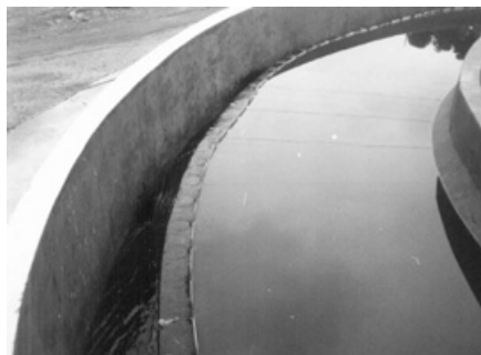
Figure 27.19. Effluent collection device (plate with V-notch weirs) Source: Nova Vista WWTP, Itabira, Minas Gerais, Brazil
