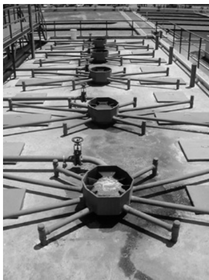
Figure 27.17. Influent distribution structure in a rectangular reactor (source: Ipatinga WWTP, COPASA, Brazil)
