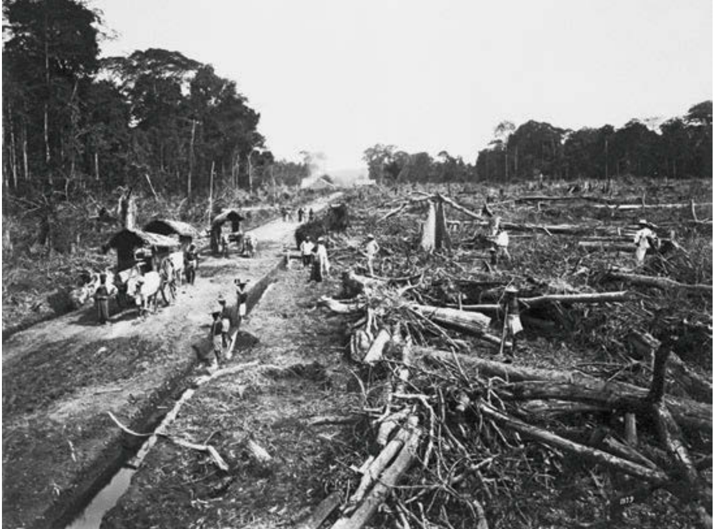
228 Cleared forest and drainage canal under construction at a tobacco plantation. Sumatra (Indonesia), around 1900.
