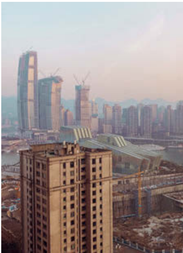
75 Construction site of Raffles City Chongqing, landmark architecture on the Yuzhong peninsula, completed in 2019.
