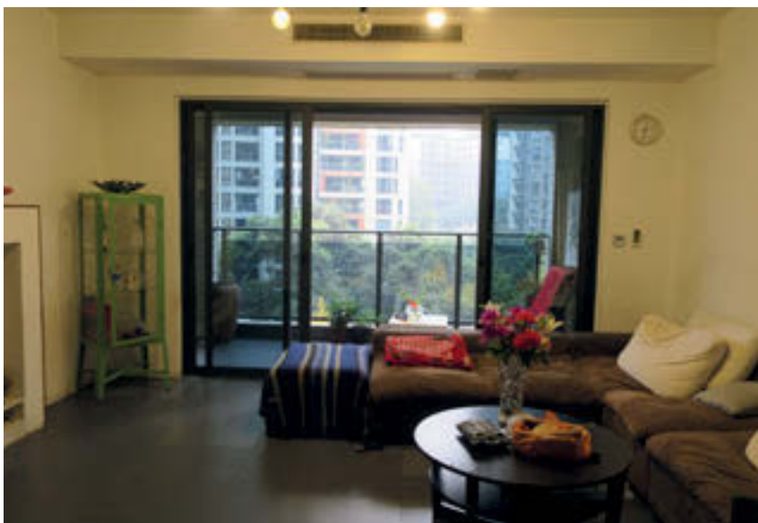
93 Example of an in-ceiling built-in air-conditioning system (top center behind the light bulbs) in the living room of a high-rise apartment in Chongqing.
