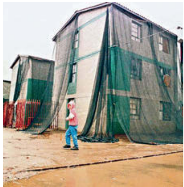
45 COPEVA houses, wrapped in plastic during rainstorms given their deficient construction and leaking exterior walls.
