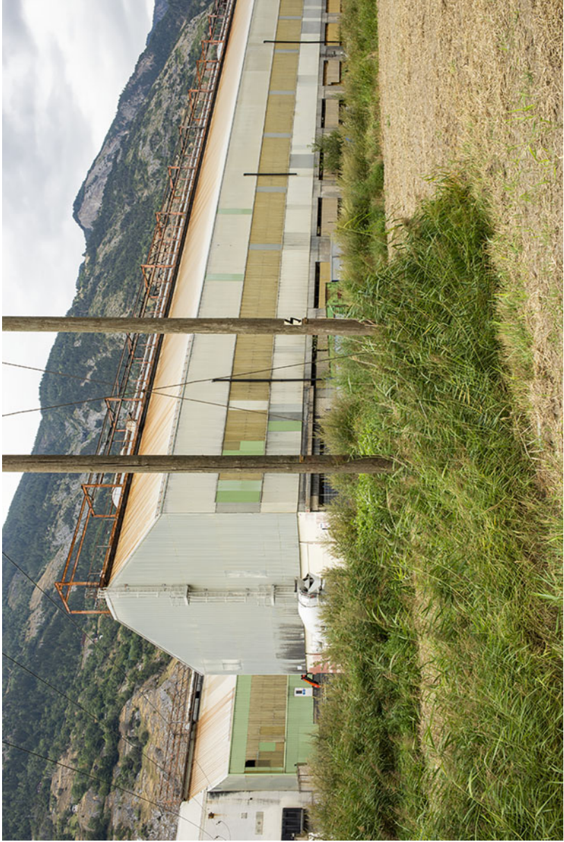
Fig. 7.91 The former electrolysis halls, now empty and derelict, in close contact with agricultural land
