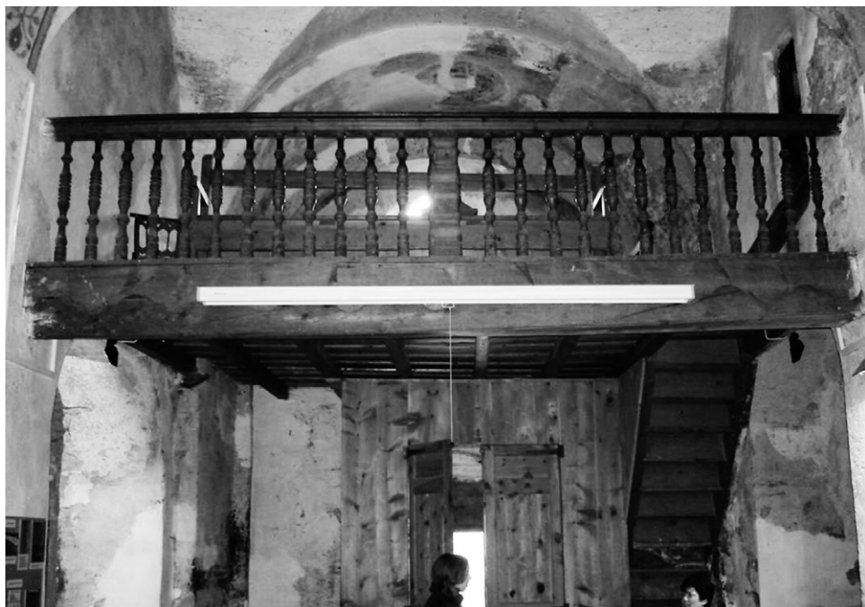
FIGURE 2 : Cor: elevated part on a higher floor inside the nave. 12. 11. 2006. Photheadographer : Izar Martínez. Place: Church Sant Pere de Sorpe.
