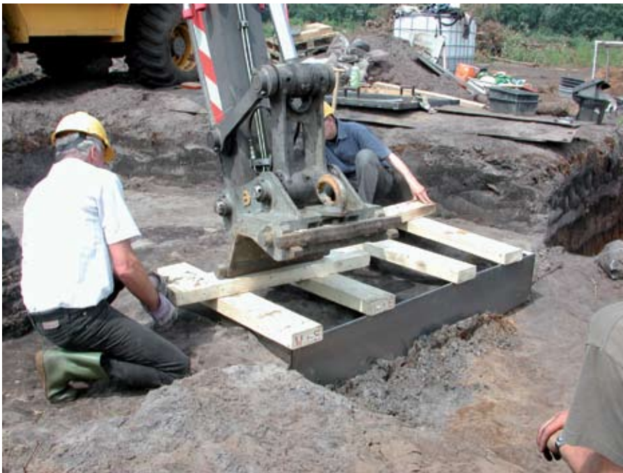
Fig. 8.4 The steel container is pushed into the soil. Figure by Restauratieatelier Restaura, Haelen.
