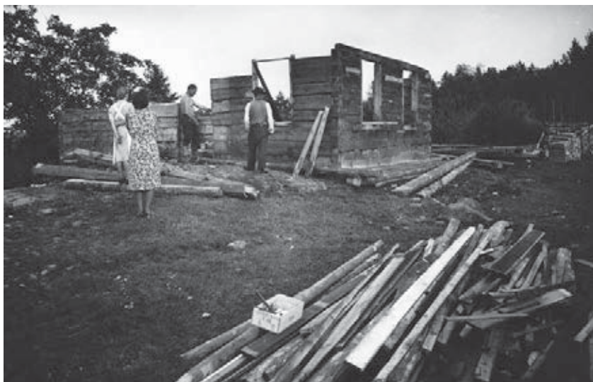
A Finnish owner rebuilds his house on its original place, Kurkijoki 1941–1944. It was a real surprise for the Soviet settlers in 1945 that houses moved during the Soviet period were brought back to their original place by the Finns. (Photo: Kurkijoki-säätiö)
