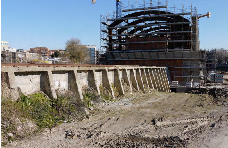
Figure 10.2 Engineering school under construction on the grounds of the old ship shute, Vasca Navale. Architect Professor Andrea Vidotto. Photo: Ola Wetterberg, 2010
