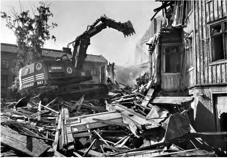
Figure 3.3 The stigmatisation of the urban vernacular historic buildings in the imaginary geography of sanitisation. The idea of urban sanitisation gradually radicalises when, during the mid-twentieth century, the claims on renewal gain political power. The imaginary geography of sanitisation builds upon the two parallel imaginary geographies (focus on monuments and/or historical buildings in the urban periphery) and develops it into making Haga appear as the epitome of ‘old-and-ugly’. The city’s planning manager, Tage William-Olsson, in a 1943 daily newspaper interview states that ‘Haga lacks the idyll found in for example Majorna [that is, Gröna Gatan] where there are several preservation-worthy buildings. From a cultural-historic point of view I cannot find any reason to keep away from sanitisation of Haga [...] The proper and rational thing to do is to demolish the old hovels and build new.’ [ Haga saknar sådana idyller som exempelvis Majorna där det finns åtskilligt man vill bevara. Ur kulturhistorisk synpunkt kan jag inte finna att det finns något som hindrar en sanering av Haga. [...] Det enda man kan göra i Haga är att rationellt riva ned de gamla rucklena och bygga nytt. (Stadsplanechef Tage William-Olsson, in Göteborgs-Posten 1943, “Sanering av Haga ....”) Photo: Lars Mongs
