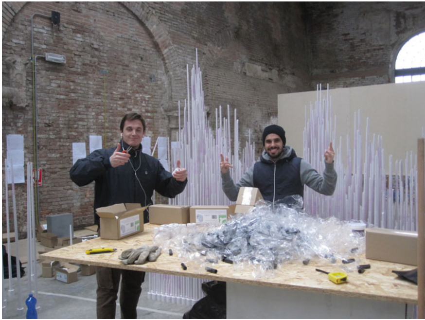
Fig. 8.8 Townsley J. Installing Till Rolls at the Venice Arsenal, Arte Laguna Prize (2013), Copyright © Jill Townsley, reproduced with permissions
