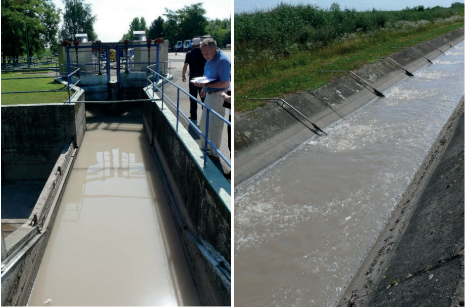
Figure 13.2 Channel connecting the primary and secondary treatment at WWTP Varaždin (photos: Meijer S.C.F.).
