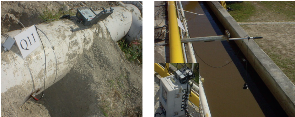
Figure 12.3 Flow measurements in closed full tubes (left) and in an open canal (right).
