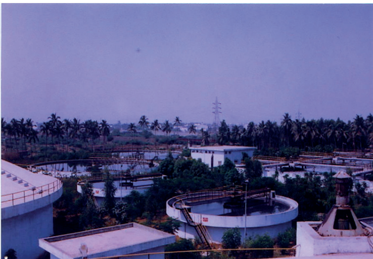
Figure 8.1 Wastewater treatment plant in Anjana.
