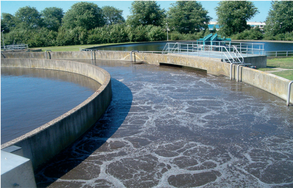
Figure 3.12 Activated sludge tank at WWTP Haarlem Waarderpolder with anoxic inner ring and outer aerobic ring and overflow to secondary clarifier (Photo: Brdjanovic D.).
