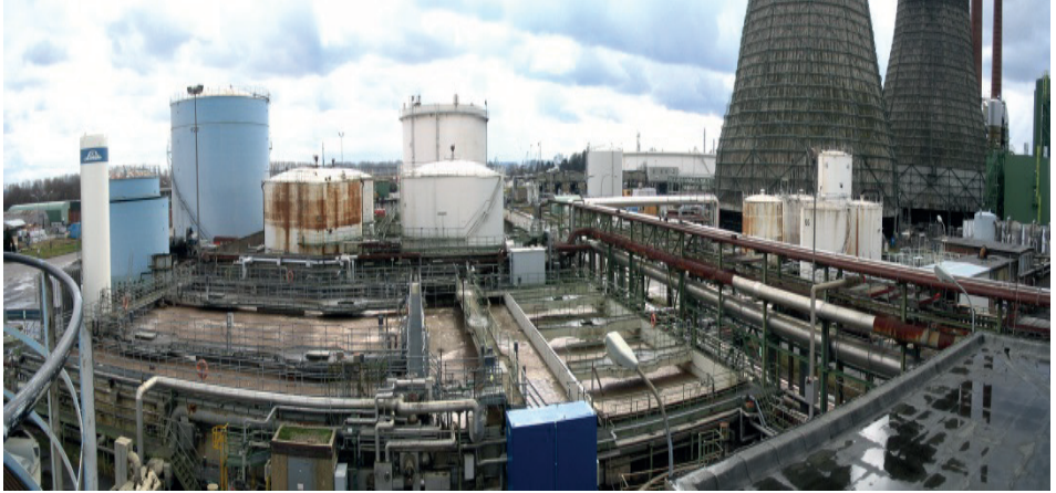
Figure 6.5 WWTP Shell Godorf oil refinery, Godorf, Germany (Photo: Pinzon A.).
