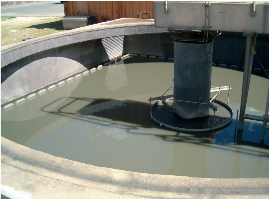
Figure 11.5 Old WWTP Illidge Rd.: final clarification (Photo: Brdjanovic D.).
