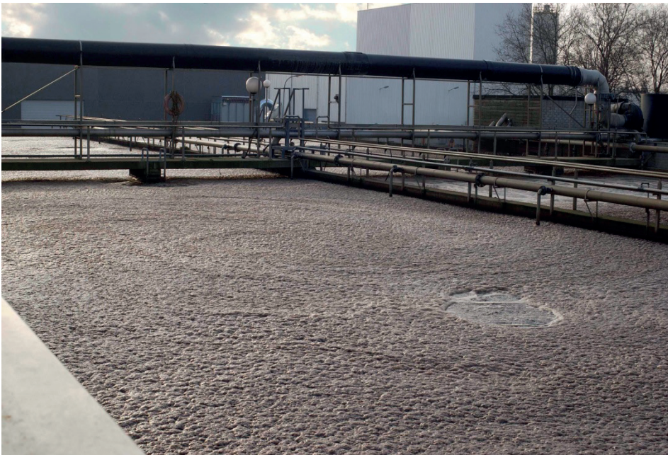
Figure 9.8 Activated sludge tank of WWTP Ecco Dongen (Photo: Moussa M.S.).
