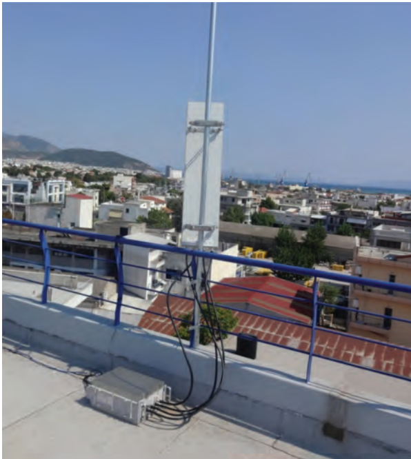
Figure 12.6 WiMAX/LTE Base Station in NITOS testbed.
