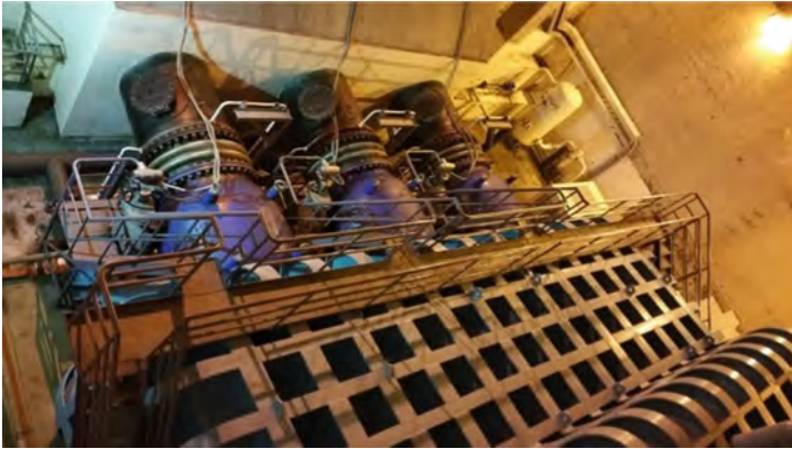
Fig. 8. Filling valves of F/E system
