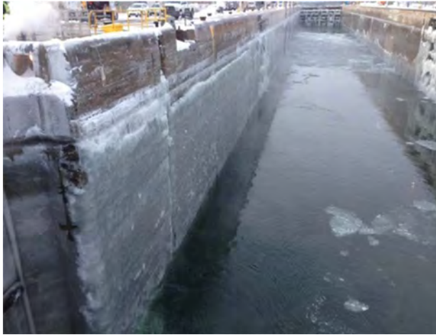
Fig. 1. Ice buildup on the lock wall surface
