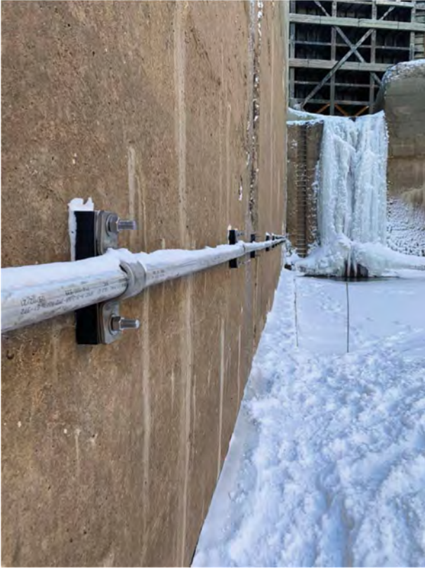
Fig. 14. Example of manifold attachment to lock wall at Upper Beauharnois
