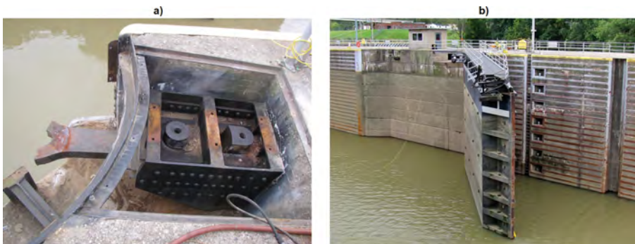
Fig. 6. Markland Lock gate failure: a) anchors of sunken leaf; b) upright leaf forced off its position, photos by USACE
