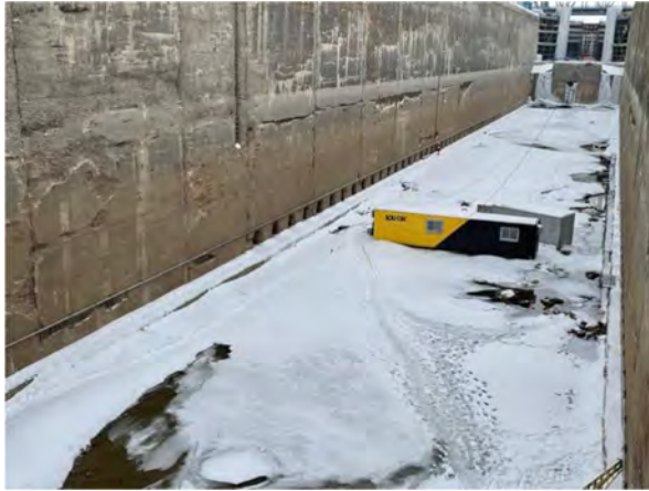
Fig. 16. Installation of one of a pair of longitudinal bubblers at the Upper Beauharnois Lock 4 in Quebec, CA. Note the installation location above the filling ports along the bottom of the lock.
