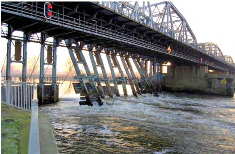
Fig. 7. Damage to Grave Weir after ship collision, photo by Rijkswaterstaat
