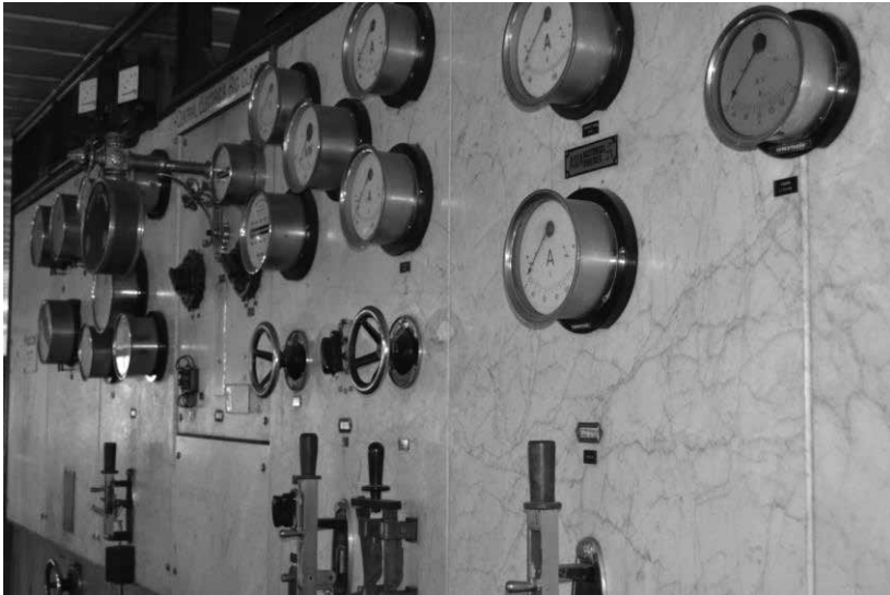
Figure 4. Corumbataí power station instrument and control panel (1925)
