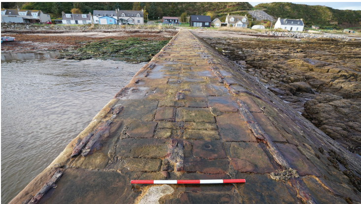
Figure 3.4 Rockfield Pier: metal strapping to seaward end. Photograph by Hilary Wyatt 2022.
