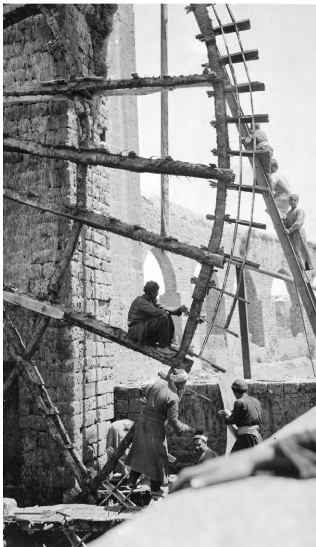
Figure 7.5 Carpenters repairing waterwheel at Hama, Syria. See letter of 13 May 1933. Olga Tufnell archive, Palestine Exploration Fund. Courtesy of the Palestine Exploration Fund.
