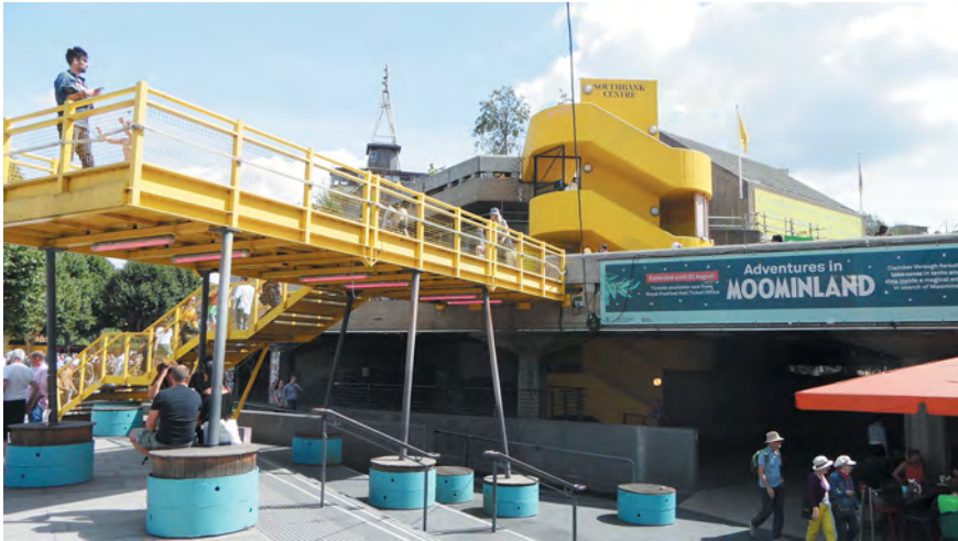
Figure 35: Responding to changing requirements. Improvised retrofitting of circulation at the Southbank Centre, London 2017
