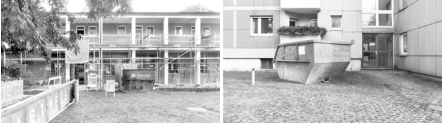
Figure 89: Parkstadt Bogenhausen, container for private refurbishment works in one of the tower blocks, Buschingstraße, Munich 2017
