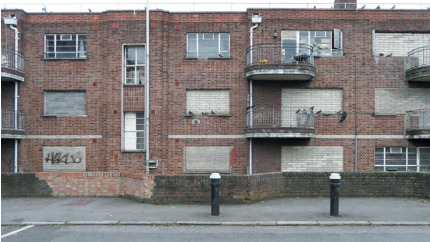
Figure 17: Obsolescence and creative destruction at work in Haggerston, London Borough of Hackney. The Kingsland Estate, built in 1949, is prepared for demolition after the majority of the residents voted in favour of urban renewal in 2007. East London 2013
