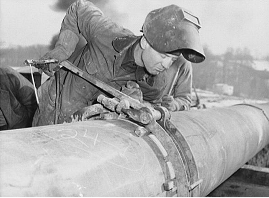
Pennsylvania section of the war emergency 24-inch pipeline to carry oil from Texas fields to eastern refineries, completed in July 1943. Willis Garner about to tack weld a section of pipe. Source: Library of Congress, Prints & Photographs Division, FSA/OWI Collection [reproduction number LC-USW3-015067-D (b&cw film neg.)].
