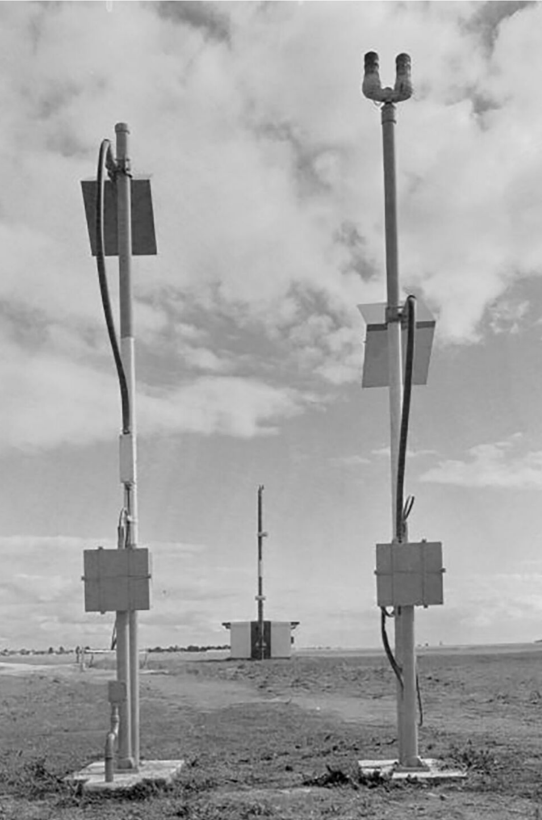
7.2 Distance measuring equipment, 1957 (Photograph Wolfgang Sievers; National Library of Australia)
