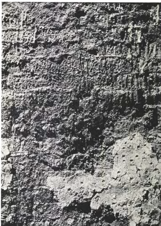
b. The staircase wall (room 3) showing vitrified brickwork: on the lower plaster is visible the finger-print keying for the intonaco
