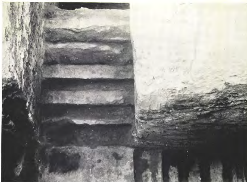
a. Room 10, looking down on the first and second flights of the newel staircase
