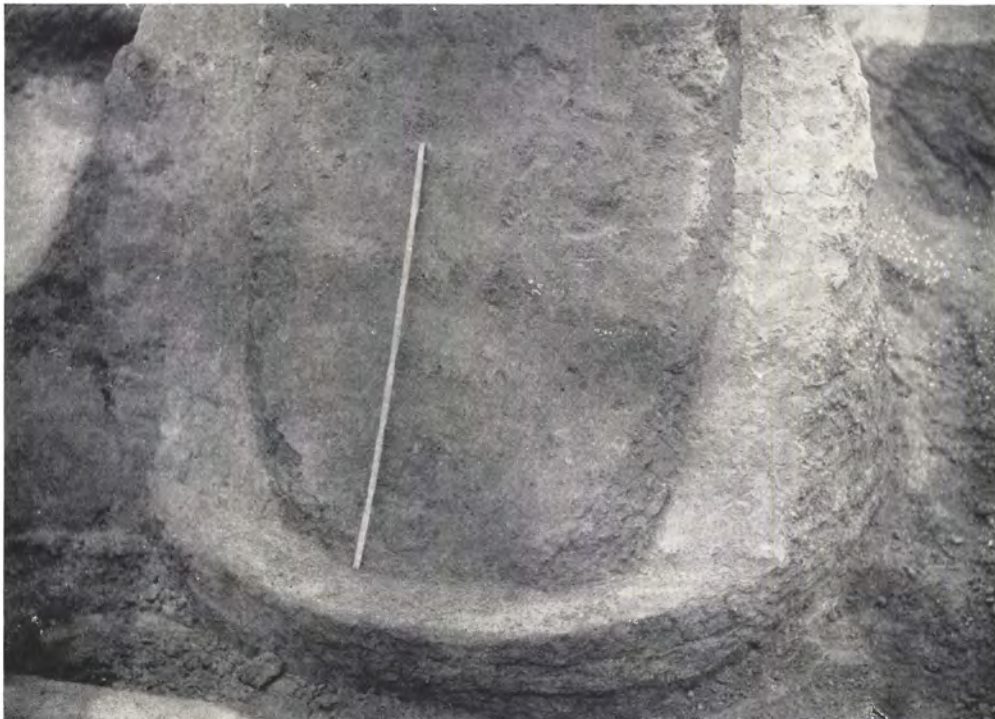
b. Section of column B, showing the new brickwork let into the old
