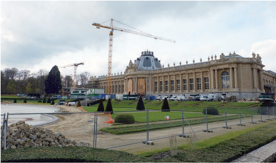
Fig. 4. A view of the Royal Museum for Central Africa (RMCA), still under construction, Tervuren, 2013
