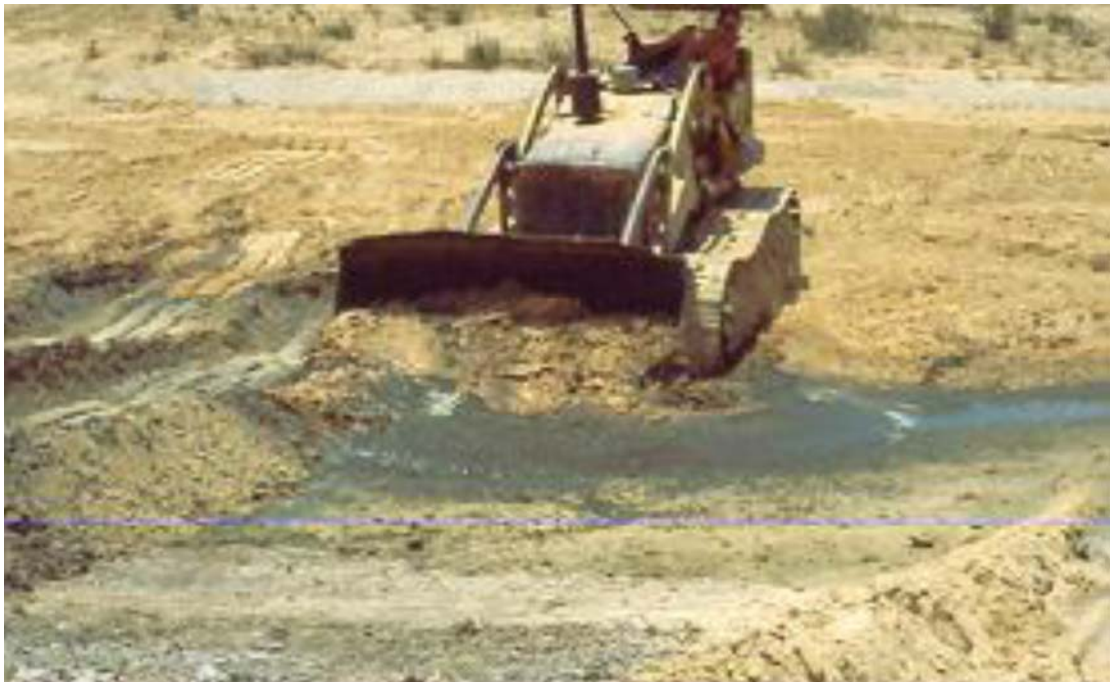
Figure 1.46 Photo of cleaning of an infiltration basin with mechanical equipment, to recover its infiltration capacity
