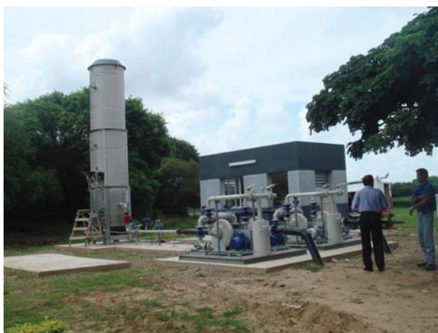
Figure 1.58 The biogas flaring system serving plants N2 and N1
