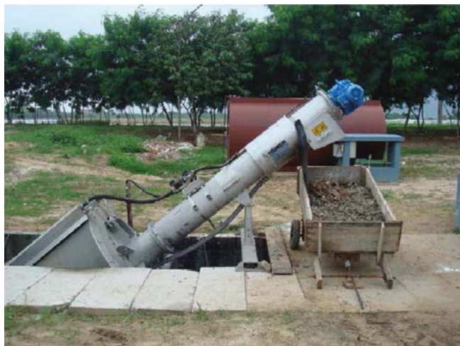
Figure 4.14 A small diameter drum of a rotating micro screen unit functioning as a pretreatment unit in the industrial park wastewater treatment plant in Santa Cruz, Bolivia
