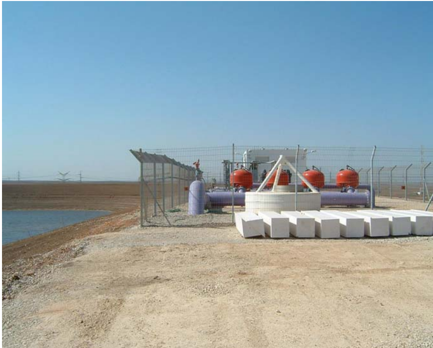
Figure 1.31 A typical disk filtration system for reservoir effluent filtration at the Kfar Menahem reservoir
