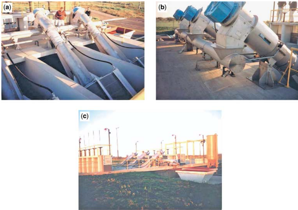
Figure 4.15 A preliminary treatment plant in La Plata, Argentina consisting of 3 parallel large diameter drums of rotation micro screens
