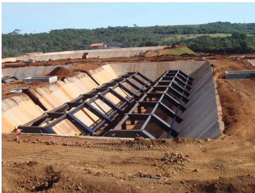
Figure 1.8 A buried UASB tank under construction in the treatment plant of the City of Uberaba, Brazil
