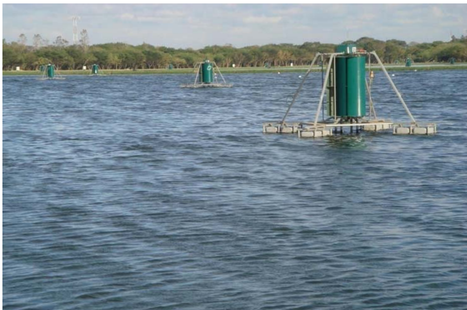
Figure 1.17 Mixers in a facultative lagoon in the N2 plant in Santa Cruz, Bolivia
