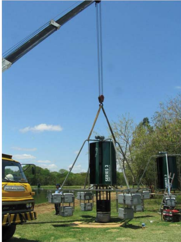
Figure 5.14 Photo of a mixer before its installation in a lagoon
