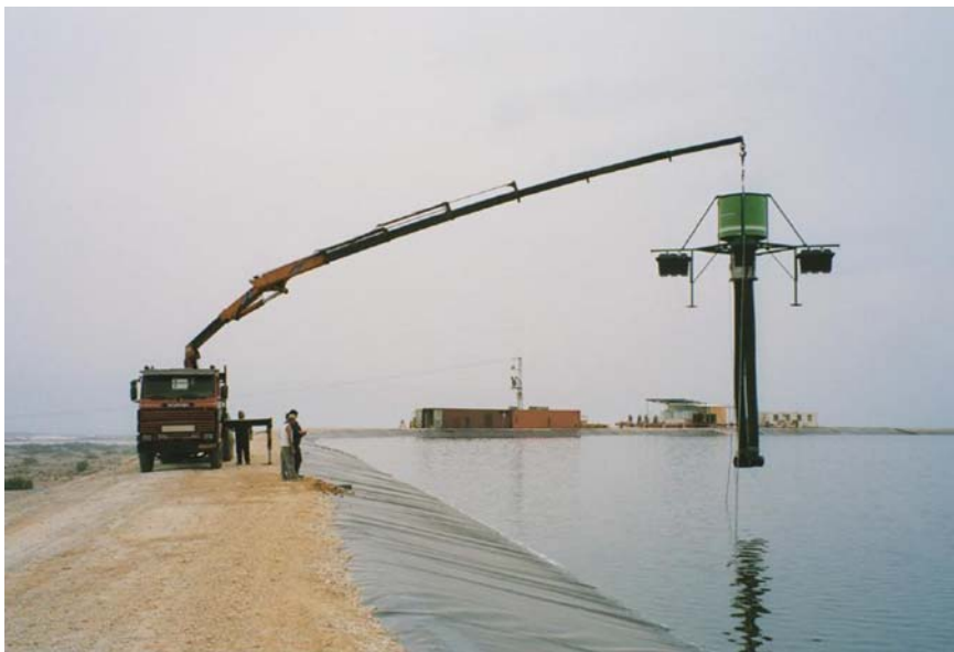
Figure 1.32 Installation of mixers in a stabilization reservoir (the Og reservoir in Israel)
