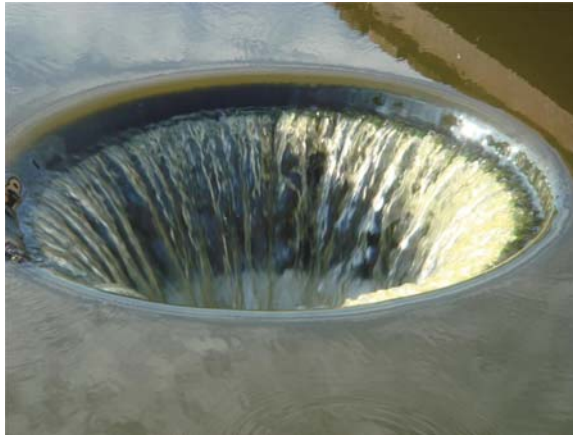
Figure 5.20 A photo of a lagoon outlet structure of the type presented in Figure 5.18
