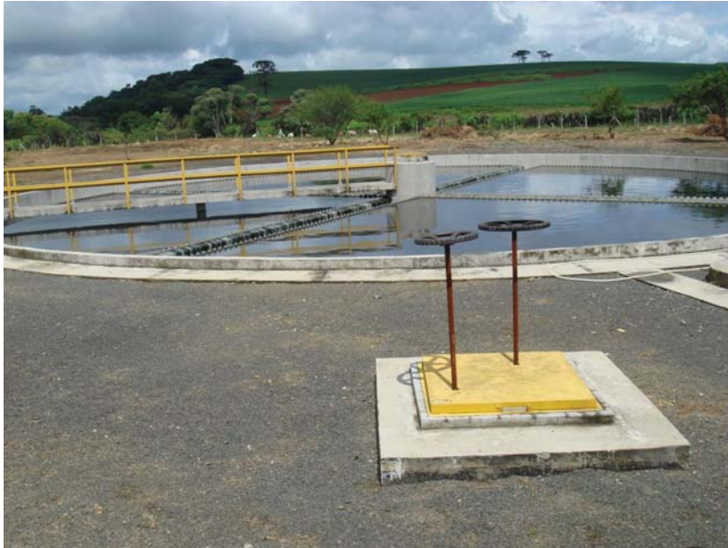
Figure 1.10 An anaerobic filter in the wastewater treatment plant of the City of Tibagi in Parana, Brazil
