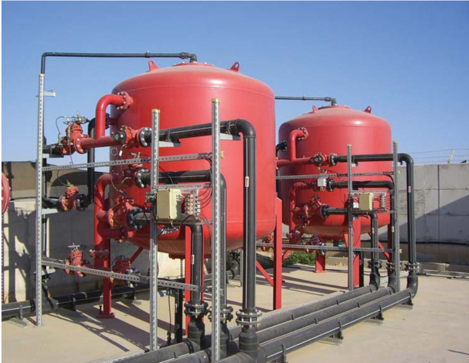
Figure 7.12 A typical sand filtration system for reservoir effluent filtration at the lehavim reservoir
