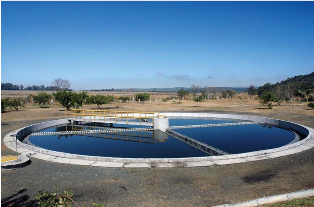
Figure 1.66 The circular anaerobic filter at the Tibagi wastewater treatment plant
