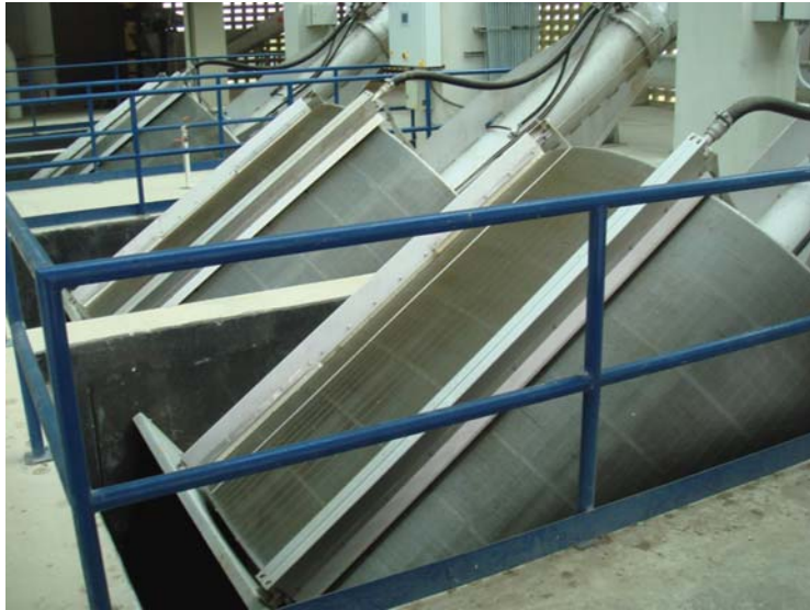
Figure 4.17 The rotating micro screen drums located inside the building of the treatment plant of Cartagena
