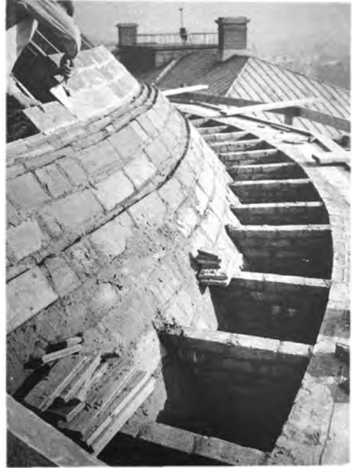
Figure 4. Construction progress image of outer dome of St. Paul's Chapel. Photograph by the author, Guastavino Fireproof Construction Company architectural records, 1866–1985, Avery Architectural & Fine Arts Library, Columbia University.
