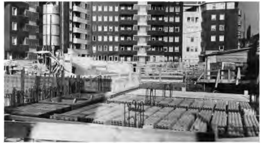
Figure 7. Centro Romana district site tower: in the foreground, the hollow floor blocks before casting concrete slab. Source: ACS, SGI collection, folder 4091–105, Photographic archive.
