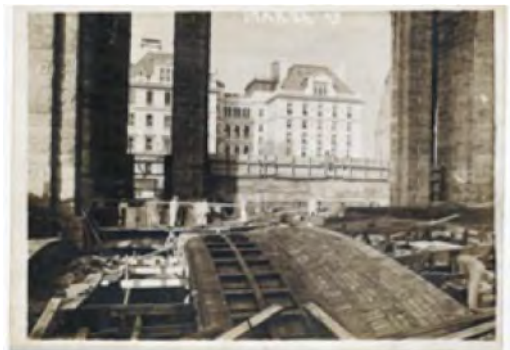
Figure 3. Construction progress image of the crypts of St. John the Divine. Guastavino Fireproof Construction Company architectural records, 1866–1985, Avery Architectural & Fine Arts Library, Columbia University.
