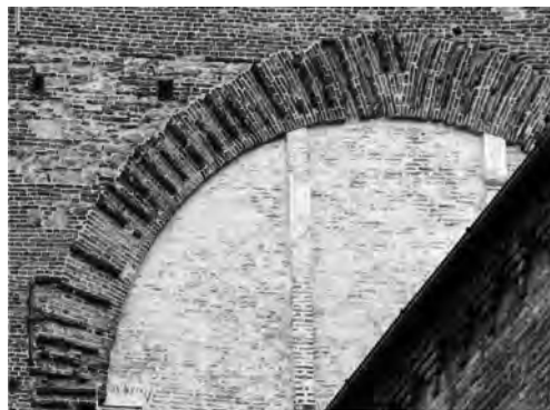
Figure 3. Example of an arch with parallel rather than radial brick courses caused by uniform mortar joints, resulting in an irregular wedge-shaped closure (Bologna, Santo Stefano; author).
