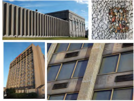
Figures 12, 13, 14, and 15 (clockwise). Above: 1004 Chouteau Ave., detail photograph with aggregate and epoxy coating. Below: Sheraton Hotel, Westport Plaza, with detail photograph showing prevalent caulk detail. (photo credit: author).
