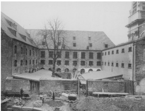
Figure 3. Demolition contractor Guillaume Sauvage had 120 days to demolish the former Minimes Prison in Brussels in 1922. Collection Comité d'Etudes du Vieux Bruxelles © KIK-IRPA Brussels .
