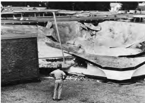
Figure 2. The collapsed shell structure of the Tucker High School (Richmond Times Dispatch).
