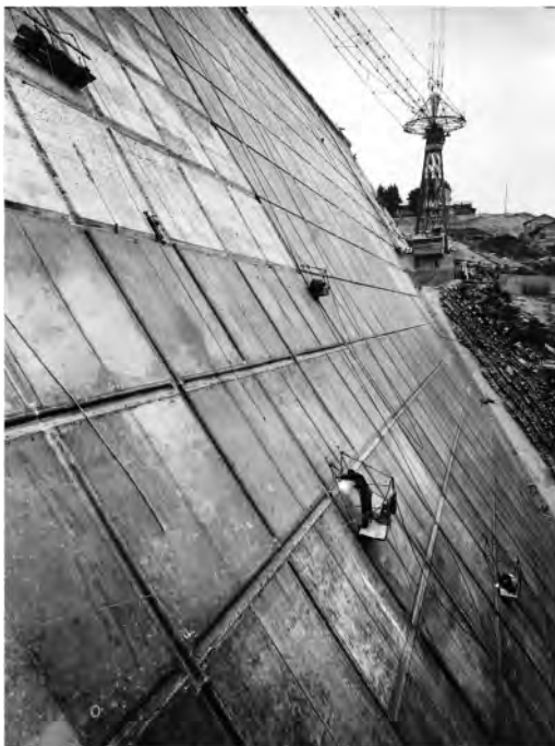
Figure 9. Platani Dam in concrete blocks, 1953–55. Construction site view of the upstream face (SIXXIdata: Claudio Marcello Private Archive).
