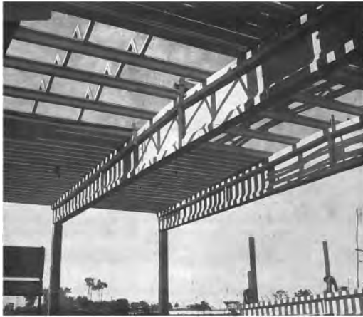
Figure 6. The Cotton warehouse in construction, with the prestored beams and the hollow slabs (Rêgo 1951a).
