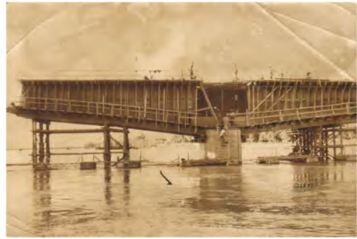
Figure 5. The Bridge over the Euphrates in Fallujah. The building site – scaffolds for the cantilevers. Source: photo collection of J. Jovanović.
