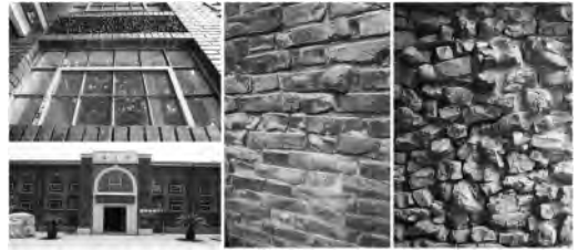
Figure 10. Clinker bricks produced in the SBTC used in the Smart Memorial Gymnasium built in 1934–7 (photos by Yiting Pan 2018).
