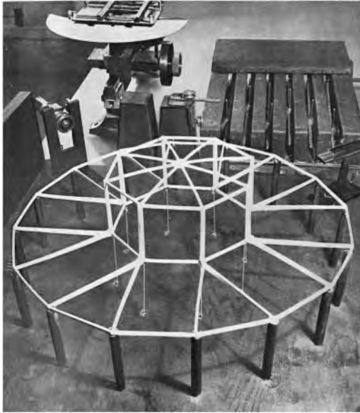
Figure 3. Life-size model built in situ. Load test for operating of the reinforced concrete cantilever slab supported by three pillars, at Hospital Clínico. Archivo Torroja, CEHOPU-CEDEX, I-ETM-095-01.
