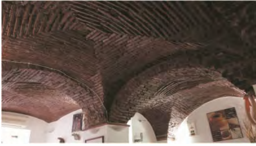
Figure 6. Winery in Borba – Groin vaults and brick arches. Source: Rosado & Reimão Costa 2020.
