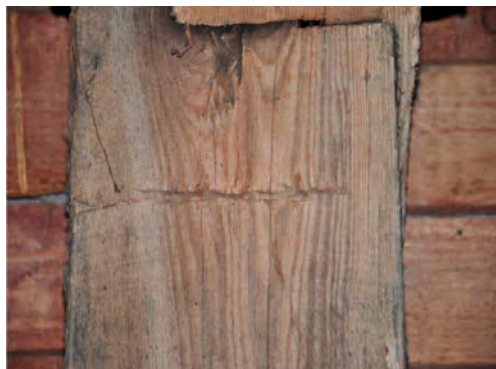
Figure 10. Toruń, parish church of St John, roof structure over the south aisle, rafter with traces of transverse cuts attesting to the initial treatment with an axe.
