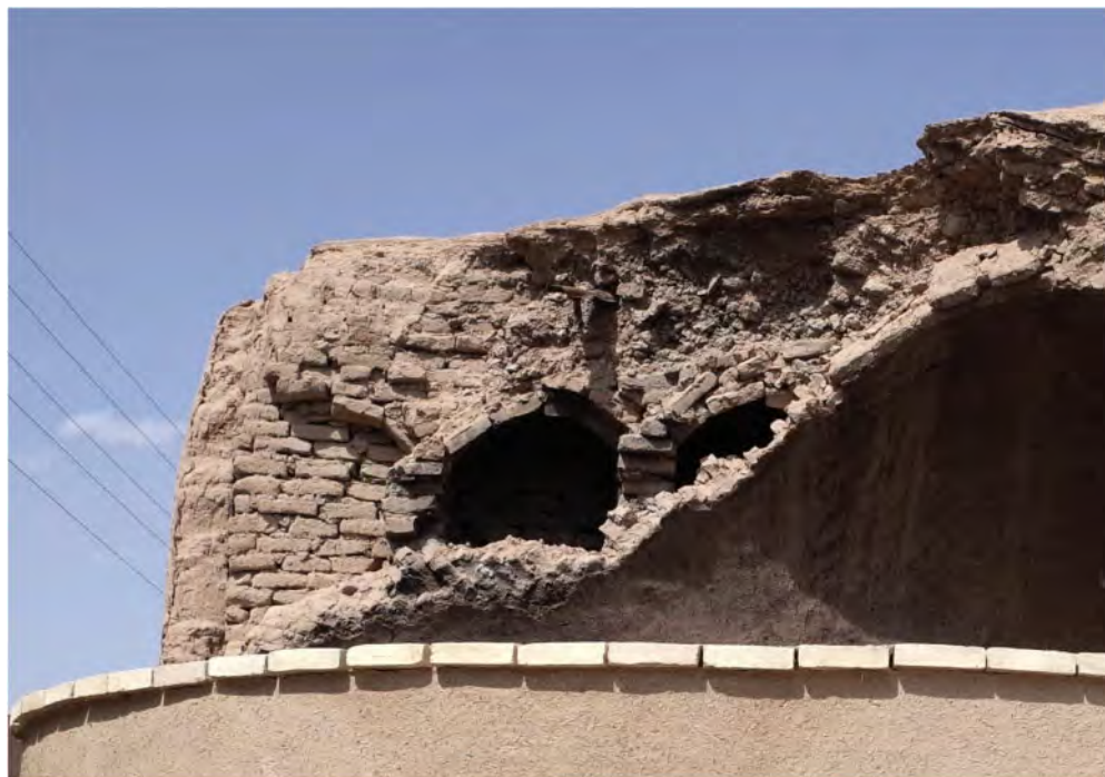
Figure 8. Small timbrel vaults lightening the weight off the groins of a larger ruined vault in Yazd.
