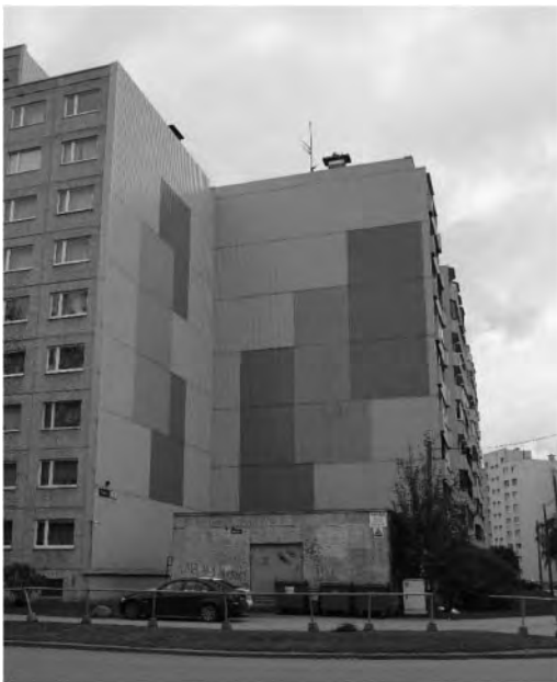
Figure 6. The end wall of an insulated apartment building covered with colourful profile metal sheet.
