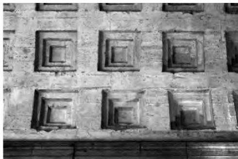
Figure 12. Palazzo Venezia, Rome. Coffered brick barrel vault of the vestibule (author). Note dislocated coffers shifted laterally with respect to the row below.
