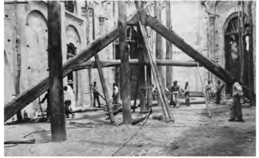
Figure 5. Xinjiang Cathedral, carpenters lifting a roof truss in the nave, 1937 (© Het Utrechts Archief, 1224, 291/45).
