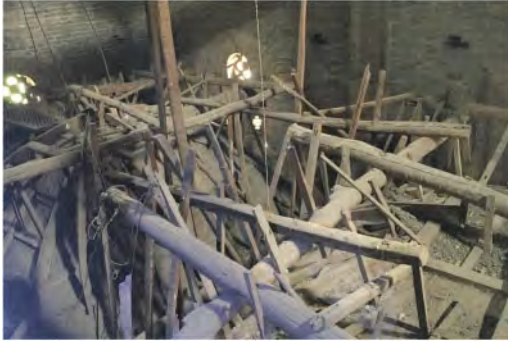
Figure 10. Xinjiang Cathedral, Bishop's Chapel, east side of the nave, space and structure above the vaults (© THOC June 2019).
