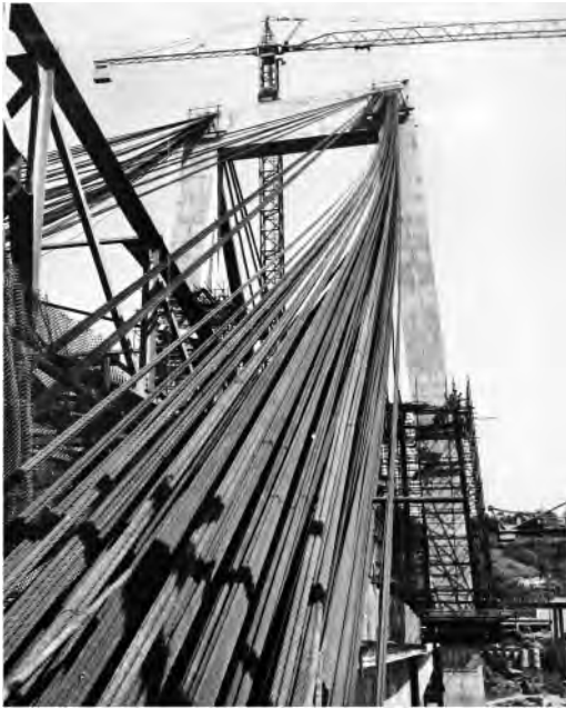
Figure 4. The bridge on the Polcevera River in Genoa. Pole 10 under construction, detail of the tie-rod cables, 10 October 1966 (SIXXIdata: Archives of the Condotte Company).
