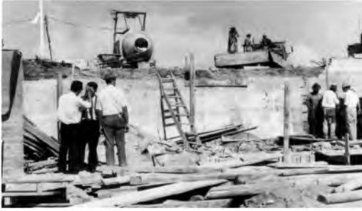
Figure 7. Ocean swimming pool, construction of the southern area (Mota, 1872; Centro de Documentação da FAUP).
