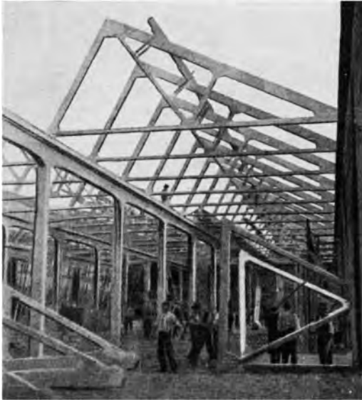
Figure 2. Assembly operation of the reinforced concrete truss girders, previously prefabricated on the ground (Santarella 1931: 346).
