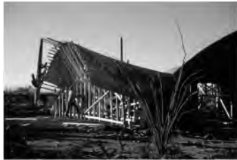
Figure 14. Formwork placement (photos by Howard Harrenstein, 1962). Tucson Historic Preservation Foundation digital collection.
