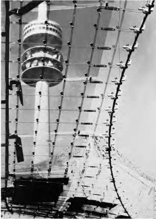
Figure 7. Olympic roof under construction. Acrylics are already mounted onto the buffers of the steel thread net. In the next step, the chloroprene rubber sheets are pressed around the edges and fixed with an aluminium frame and screws (Front cover of a greeting card with advertisement and stamps on the occasion of the Olympics 1972 from Knoll AG Ludwigshafen, unknown photographer, private property S. Brunner).
