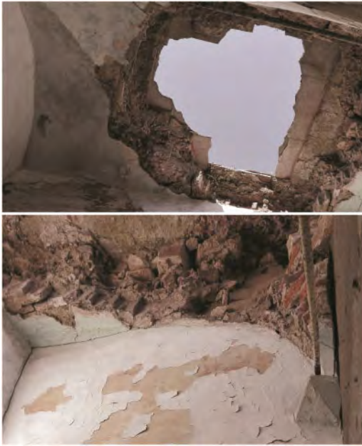
Figure 3. Roof terrace above a groin vault in Estremoz, construction attributed to c.1698. Source: Rosado & Reimão 2020.
