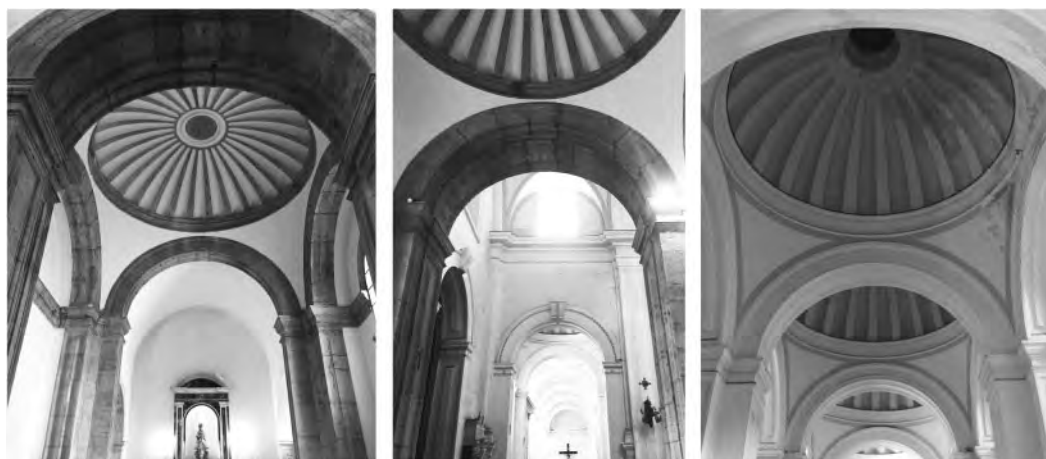
Figure 8. The piperno stone exposed at the dome intrados of the restored main chapel and the domes covering the side-aisle bays.
