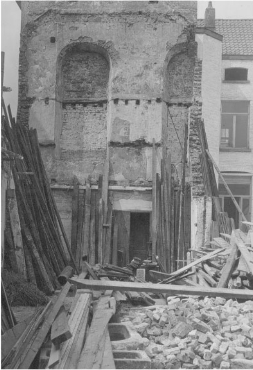
Figure 5. Sorting materials (brick, timber, blue stone) at the demolition site of Chartreux Chapel in 1905. Rue des Fabriques 1 in Brussels. Collection Comité d'Etudes du Vieux Bruxelles © KIK-IRPA Brussels.
