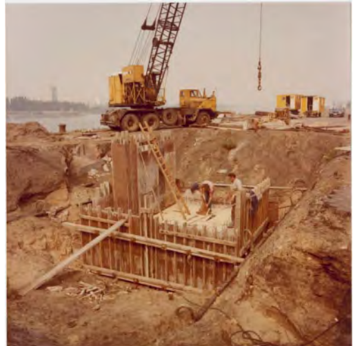
Figure 3. Water barrier Scheldt quays Antwerp, 1978. Inter-action between man, machine and technology. (Photographer unknown).
