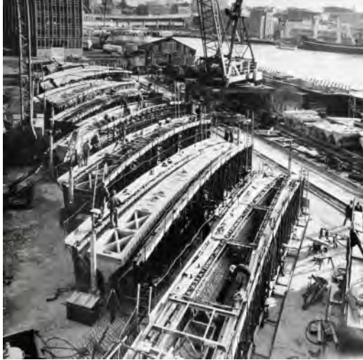
Figure 2. The rib formwork system located on the eastern side of the casting yard. Photographer: Max Dupain and Associates. Records and negative archive: un-commissioned Sydney Opera House construction photographs, 1965–1972. Courtesy: NSW State Library.
