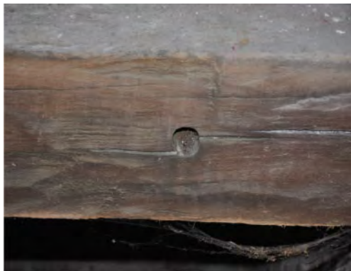
Figure 7. Toruń, parish church of St John, roof structure over the chancel, only a single opening attesting to the tying of the logs with one wedge.
