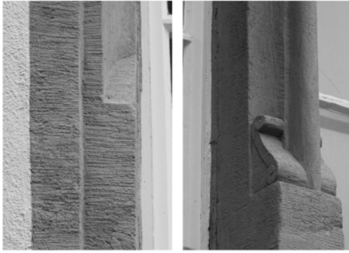
Figure 8. a (left) and b (right). Solothurn, Goldgasse 8. On the left the window jamb from 1562, on the right the jamb with volutes from 1622, both made out of sandstone (author 2020).
