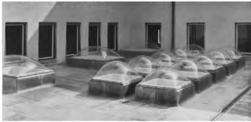
Figure 5. Roof of the Stadtparkasse Darmstadt of 1957 with two types of square shaped cupolae , single layer, screwed onto the funnel (Röhm & Haas GmbH 1957b, 32).
