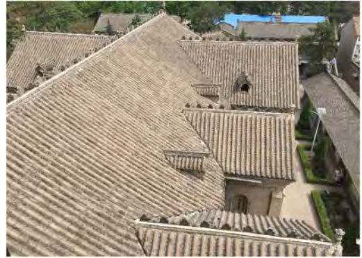
Figure 8. Xinjiang Cathedral, roof of the nave and east side chapels, from the south-east tower (© THOC June 2019).
