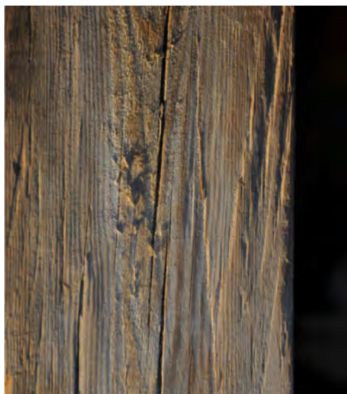
Figure 12. Toruń, parish church of St John, roof structure over the north aisle, long and slightly tilted cuts on the rafters attesting to the smoothing of the building material with a broad axe.
