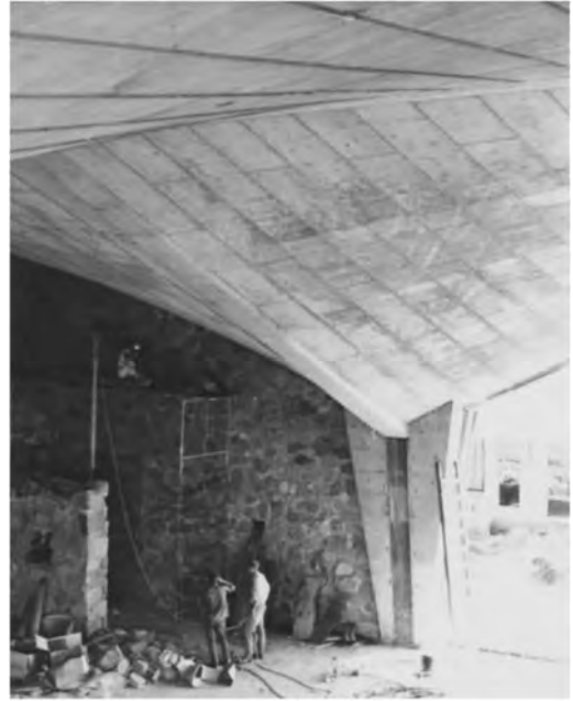
Figure 12. Interior of the hypars on the Main Church of the Annunciation Priory, Bismarck, North Dakota, USA, 1962. Marcel Breuer Digital Archive.
