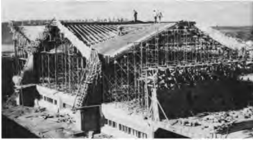
Figure 13. Construction process of the roof on the main church of the Annunciation Priory, Bismarck, North Dakota, USA, 1962. Marcel Breuer Digital Archive.
