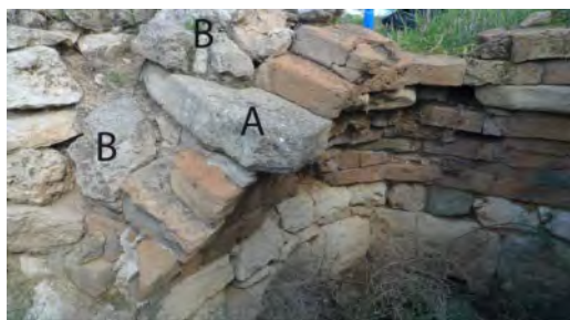
Figure 2. Detail of the brick vault. A) row of limestones set at the height of the haunches. B) rubble stone filling.
