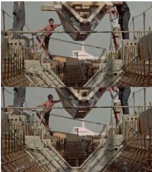
Figure 7. Images from the documentary Jørn Utzon: The Man & The Architect (2018) showing the internal formwork lowered on top of a rib-bed. Courtesy: Sydney Opera House.
