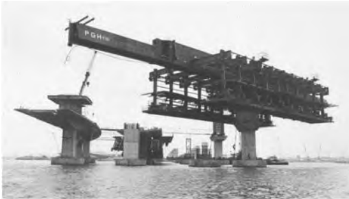
Figure 1. Third mainland bridge over the Lagos Lagoon, S. Zorzi, 1976–80 (Inco Archive, Milan).
