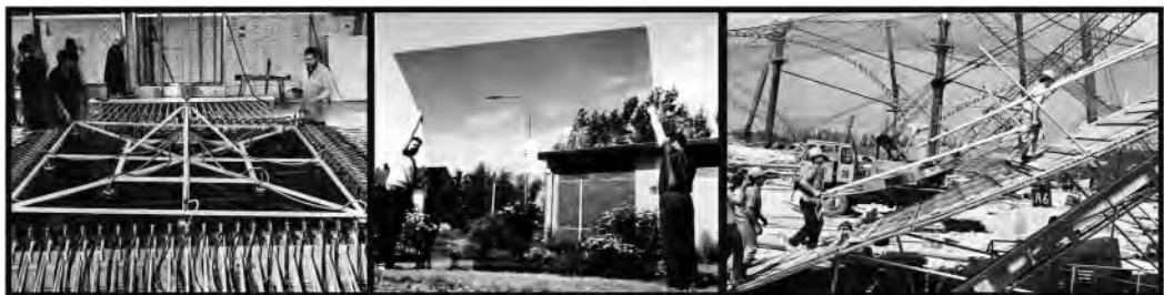
Figure 8. Left: Biaxial stretch forming of cast Plexiglas at Röhm & Haas in Darmstadt in 1970. Middle: First sheet for the roof in 1971. Right: Construction site, transport onto the Olympic roof in 1971 in Munich (Photos: Evonik Industries AG, Corporate Archives, Record Group Röhm, Photo Archives, Hanau).
