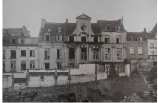
Figure 4. Window frames are taken out of the buildings before demolishing the houses on Rue Montagne de Sion. Collection Comité d'Etudes du Vieux Bruxelles © Bibliothèque artistique, ArBA .
