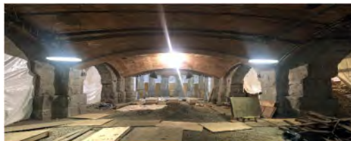
Figure 6. Tile arches and vaults in the crypt of Saint John the Divine. The arches running left to right in the photo were constructed first, followed by the doubly-curved vaults. Photograph by Derek Trelstad.
