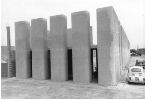
Figure 8. The construction of the envelope: internal reinforced tuff block walls (Courtesy of Franco Sargiani).
