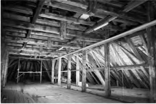
Figure 1. Catholic church St. Jakob in Cham, Canton of Zug, Switzerland. Overview over the roof truss, erected in late Summer or Fall 1784 (Gantner 2018).
