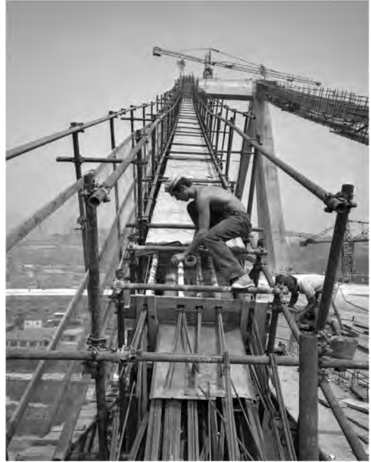
Figure 6. The bridge on the Polcevera River in construction, the stay of pile 9. Photo Mario De Biasi, August 1967 (SIXXIdata).
