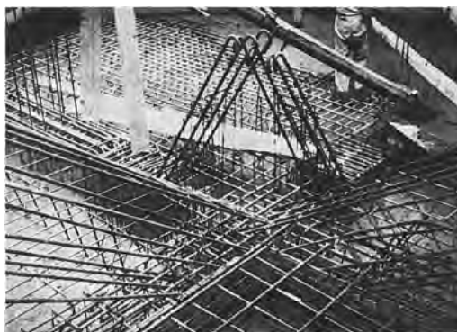
Figure 2. SNIA Viscosa Tower. Construction of the foundation plate ( L'industria italiana del cemento , 1936, 12, 329).
