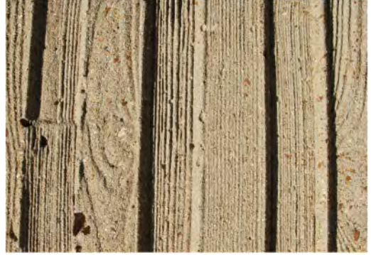
Figure 8. Pet Milk Building concrete surface imprinted with board formwork. (photo credit: author).
