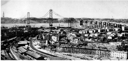
Figure 4. The suspension bridge and access viaduct under construction. Far left: the Cristo Rei monument (MOP 1966b, 28).
