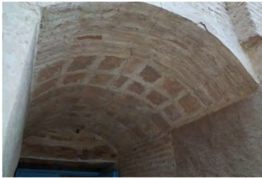
Figure 11. Timbrel vault combined with a leafed arch in the religious complex of Mahan.
