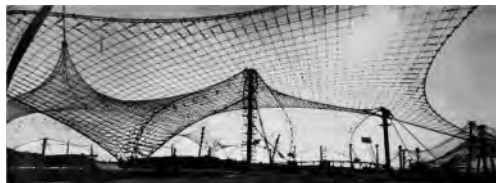
Figure 5. Pretensioned cable net construction of the roof of the swimming pool (Bach 1975, 253).
