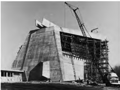
Figure 15. Construction process of lateral hyperbolic paraboloid. Church of St. Francis de Sales, Muskegon, Michigan, USA, 1966. Marcel Breuer Digital Archive.
