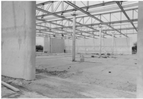
Figure 9. The steel structure contained within the wall perimeter (Courtesy of Franco Sargiani).
