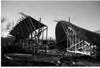
Figure 13. Formwork placement (photos by Howard Harrenstein, 1962). Tucson Historic Preservation Foundation digital collection.
