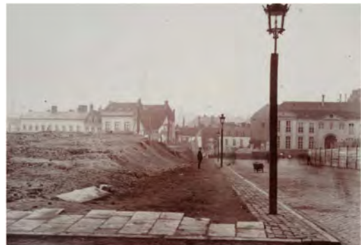
Figure 1. Vast demolition works were taking place in Brussels at the beginning of the 20th century. For instance, Rue des Douze Apôtres and Rue du Parchemin were demolished in 1909. Collection Comité d'Études du Vieux Bruxelles © Bibliothèque artistique, ArBA.
