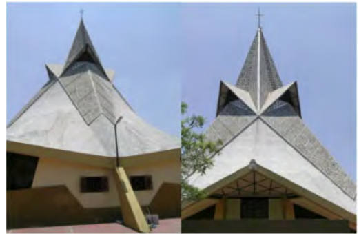
Figure 16. Exterior of the church. The support is the only point where the paraboloid sections meet (Image Moisés Escárcega).
