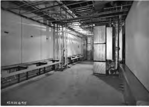
Figure 10. Horizontal piping unit above the floor.
