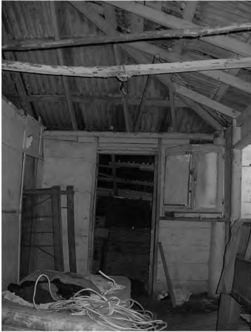
Figure 9. Interior of a casita in Planadas, an abandoned settlement in Cayey, Puerto Rico. Notice the elementariness of framing (photo by author).
