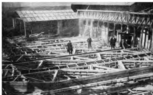
Figure 1. On-site prefabrication of the reinforced concrete truss girders within reusable wooden formwork (Santarella 1931: 346).
