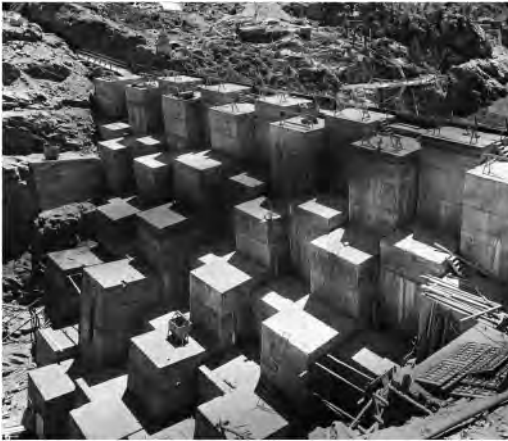
Figure 7. Concrete blocks during the construction site of the Pian Palù Dam in the Noce Valley, 1954–59 (SIXXIdata: Chiolini Photographic Archive).
