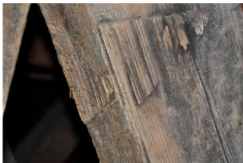
Figure 14. Toruń, parish church of St John, the north roof structure over the aisle, a triangle remaining after splitting the material at the point where the saw meets on both sides.
