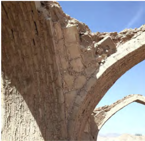
Figure 7. Springer of a timbrel vault clad with adobe bricks in the Mazdayasna funerary complex of Yazd.
