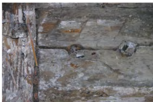
Figure 5. Toruń, 9 Marii Panny St., a bolt of the building frame with two openings, with a wedge and a tree twine in one, attesting to the rafting of wood.
