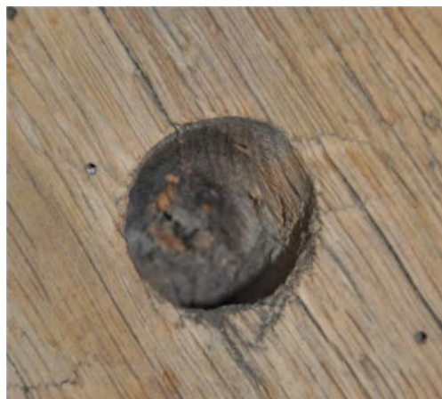
Figure 3. Toruń, parish church of St John, belfry structure, mid-15th century, a round and conical hole in cross-section opening attesting to the rafting of wood.
