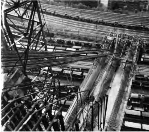
Figure 5. The bridge on the Polcevera River in Genoa. Pile 11 under construction, the saddle in the foreground, 12 May 1964 (SIXXIdata: Archives of the Condotte Company).
