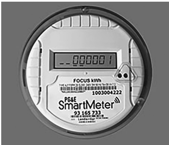
Figure 4.3 Smart meter example. (From PG&E, see http://www.pgecurrents.com/2012/06/12/pge-catches-wave-on-smartmeter-deployments/ .)
